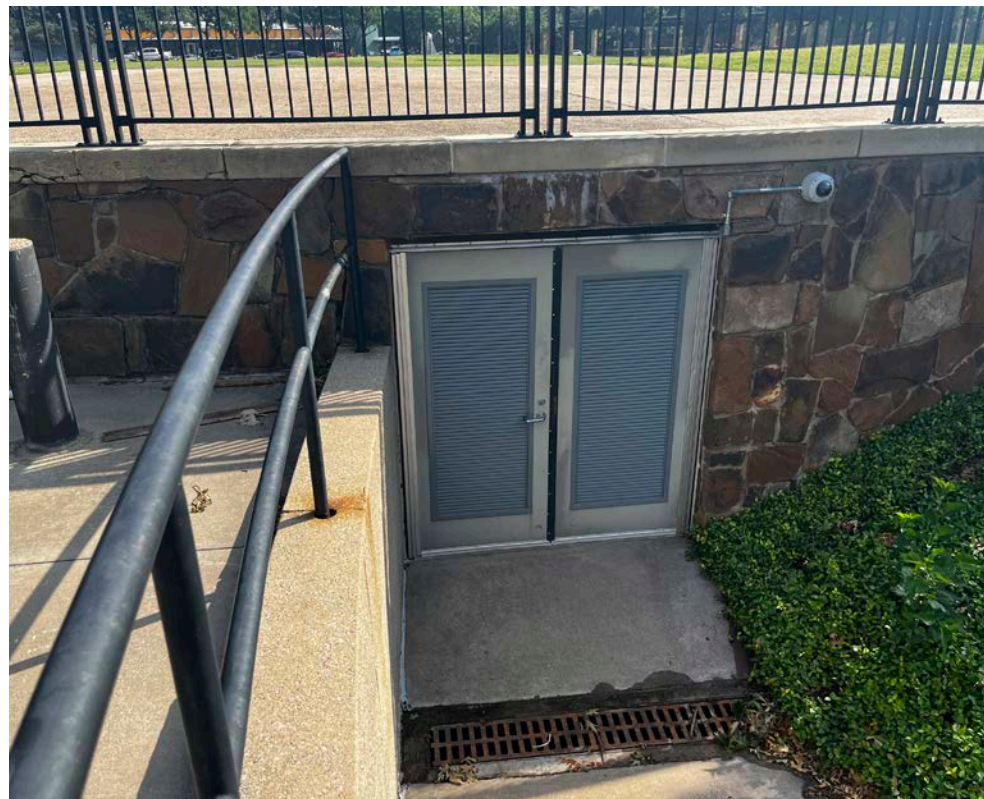
Lack of On-Site Storage
