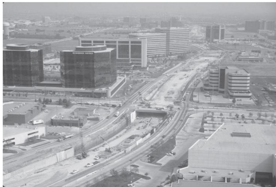
Construction of the Dallas North Tollway through Addison. The Town paid to construct the Tollway underground so that it would not cut the community in half.
