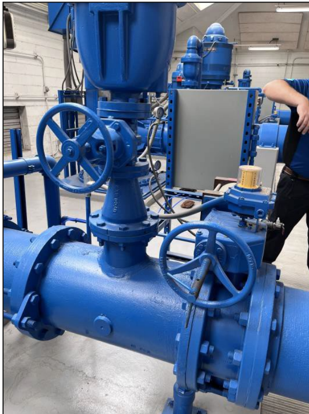
Figure 5: Photo of header
