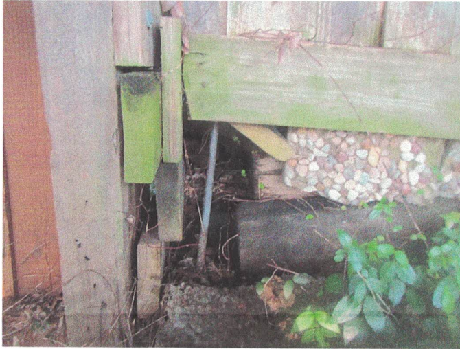
Southeast corner of 4110 Pokolodi Circle. Railroad ties are behind the veneer.
