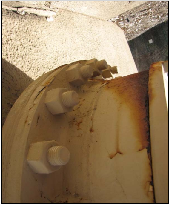
Photo 30 Overflow 1 - 24-inch Cast Iron Category: Operational
