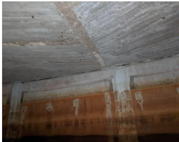
Photo No.14 – Grout Deterioration
