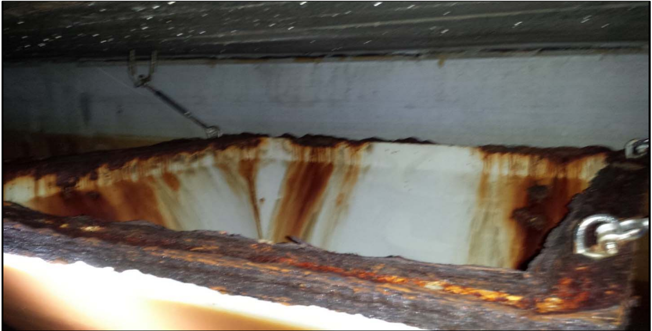
Photo 33 Overflow 1 Weir Box - 4 feet 2 inches Wide by 4 feet 2 inches Wide Category: Operational
