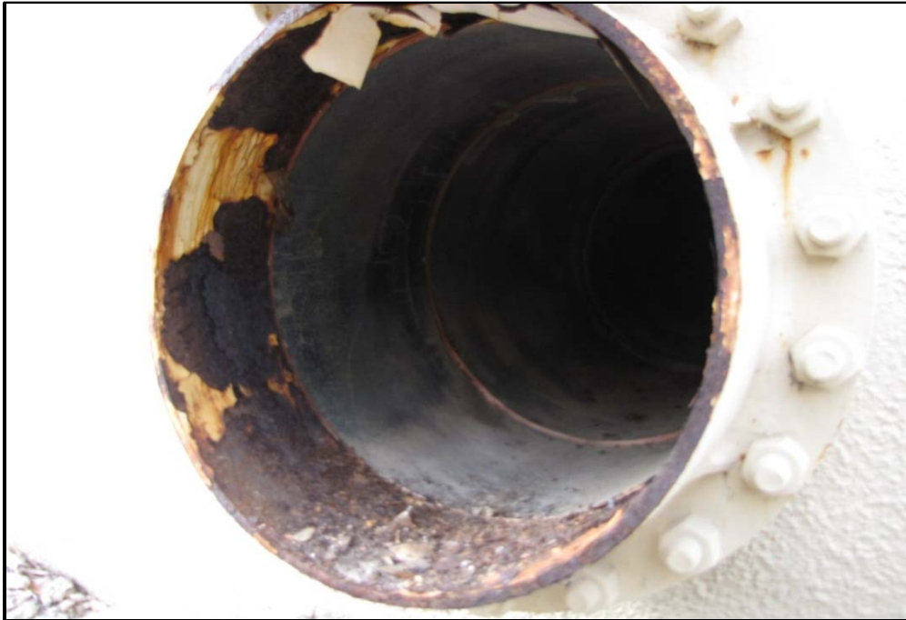
Photo 31 Overflow 1 - 24-inch Cast Iron - Interior Corrosion was Observed Category: Operational
