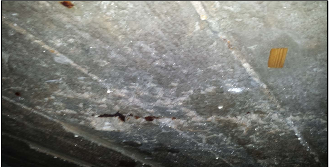
Photo 7 Interior Roof - Typical Spalling Observed Category: Structural
