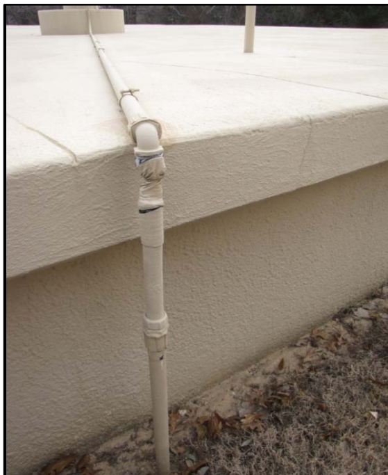
Photo 48 Electric - Formerly for Sonic Level Transmitter Category: Operational
