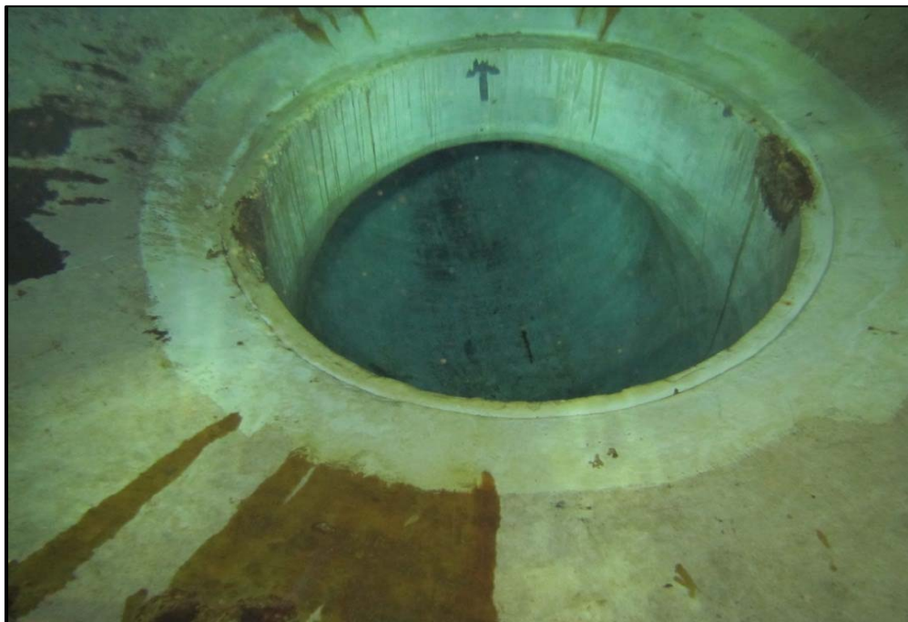
Photo 26 Outlet 1 - 42-inch Ductile Iron Category: Operational
