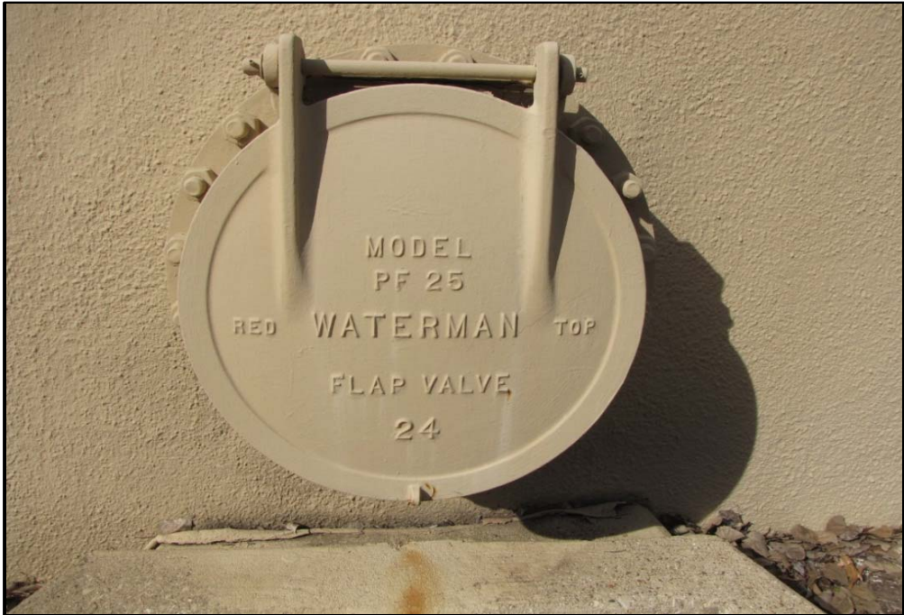
Photo 29 Overflow 1 - 24-inch Cast Iron Flap Valve Category: Operational
