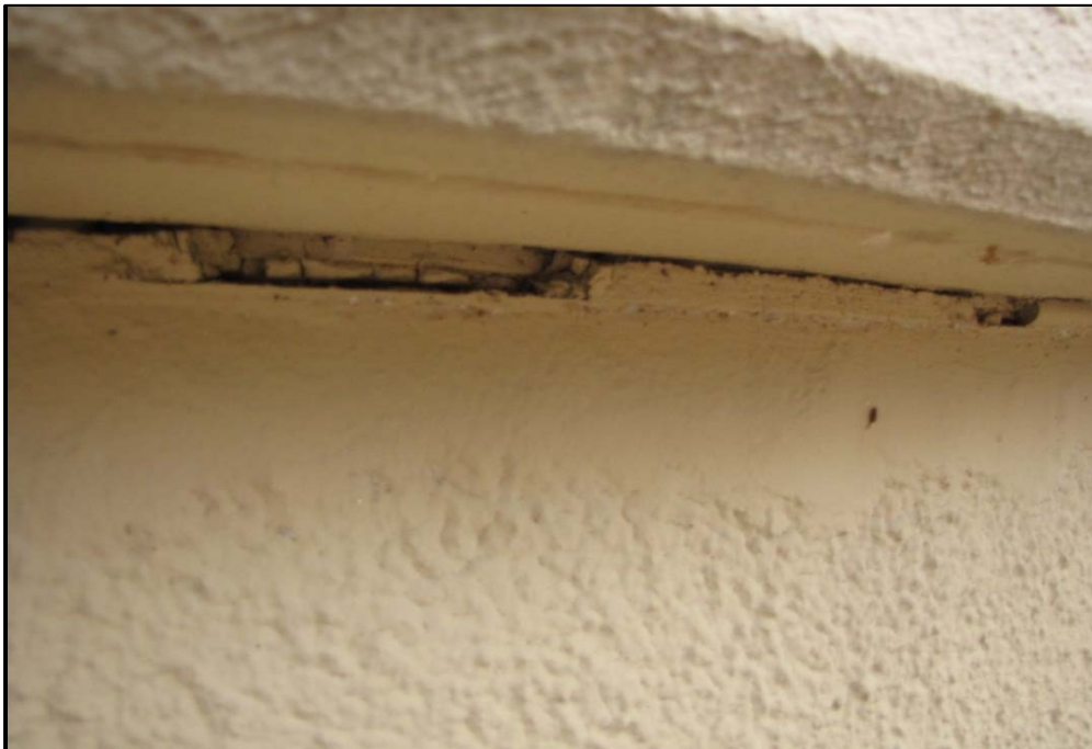
Photo 16 Shell and Roof - Observed Severe Degredation of the Joint Category: Structural
