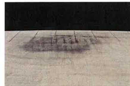
Ponding and Cracking in Exterior Roof
