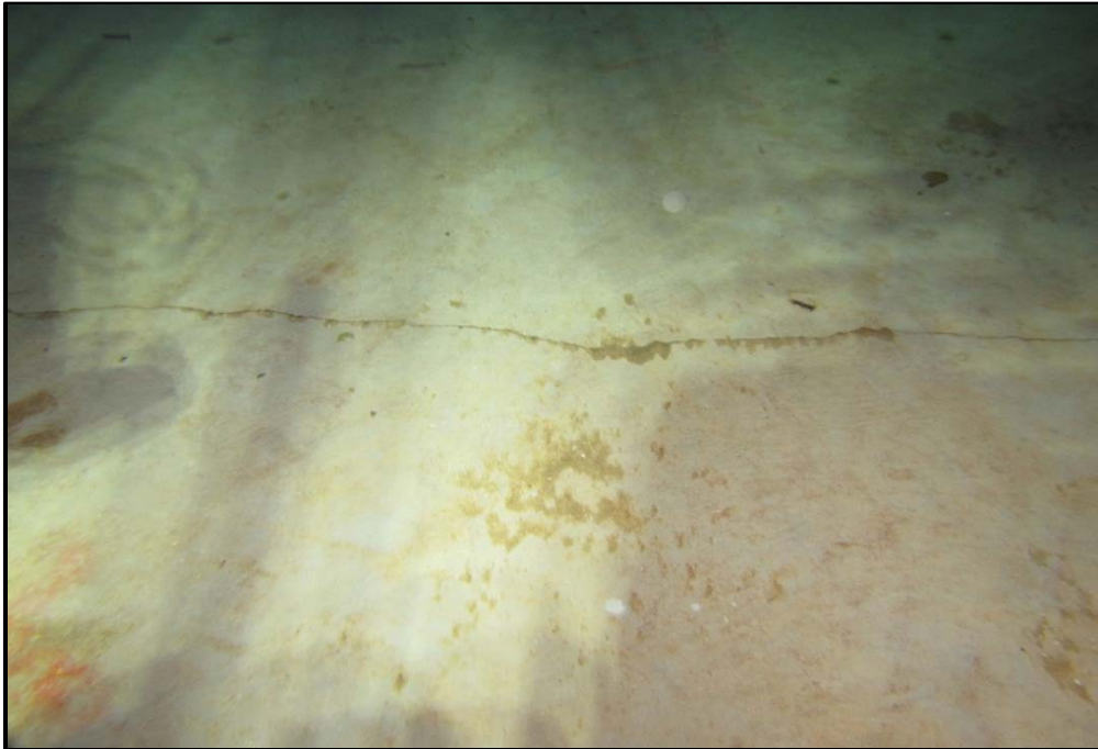
Photo 19 Interior Floor - Cracking was Observed Category: Structural
