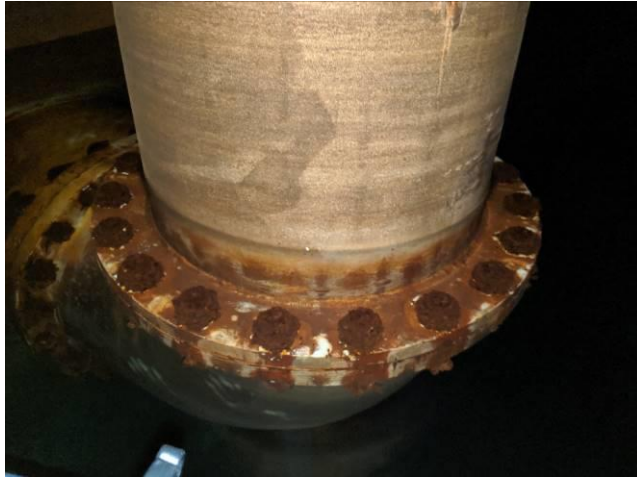
Photo No.45 – Carbon Coated Bolts (Interior)
