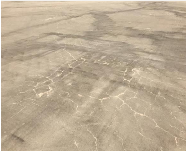
Photo No.1 - Cracking & Ponding
