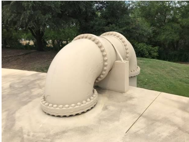
Photo No.25 – Inlet Pipe
