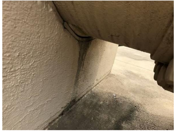
Photo No.26 – Inlet Pipe
