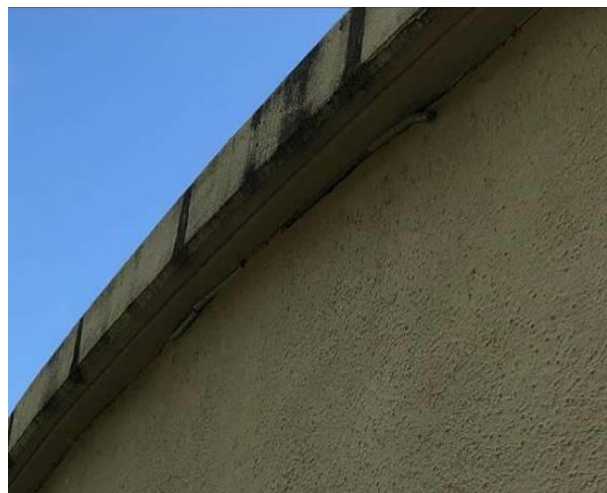
Photo No.6 - Grout Deterioration
