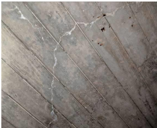
Photo No.9 - Cracking
