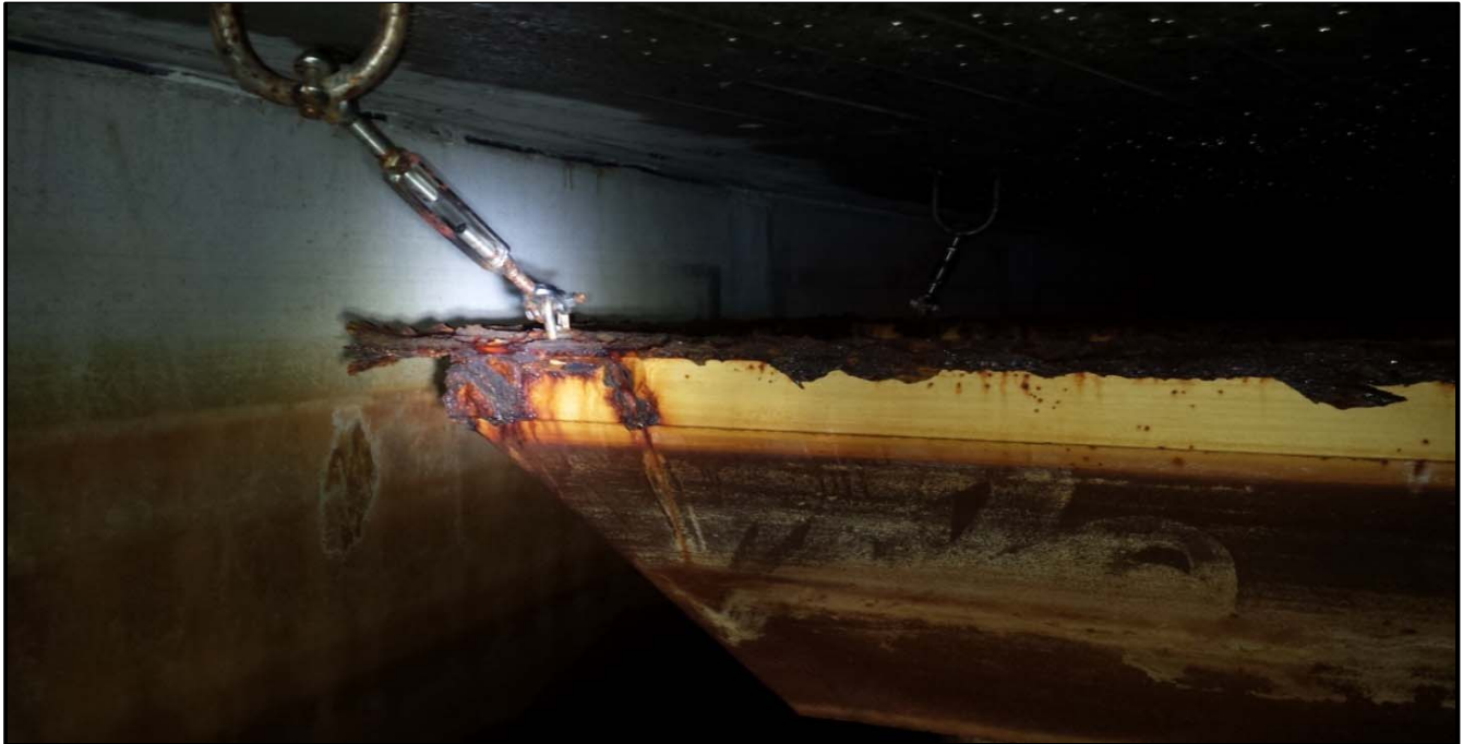
Photo 41 Overflow 2 - 1/2-inch Diameter by 6-inch Turnbuckle Category: Operational
