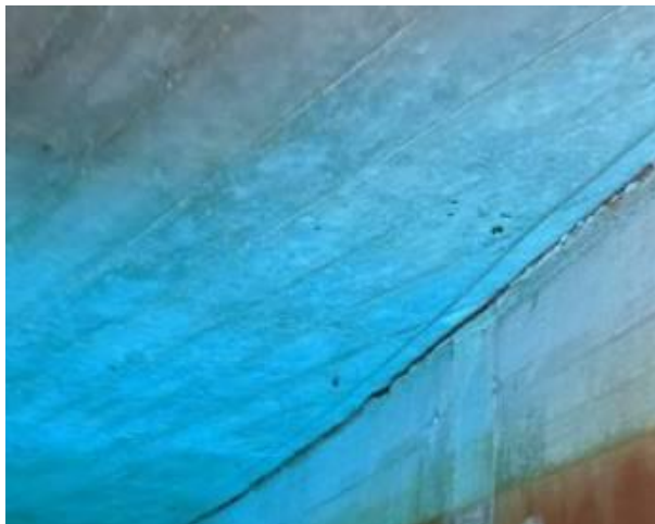
Photo No.13 – Grout Deterioration
