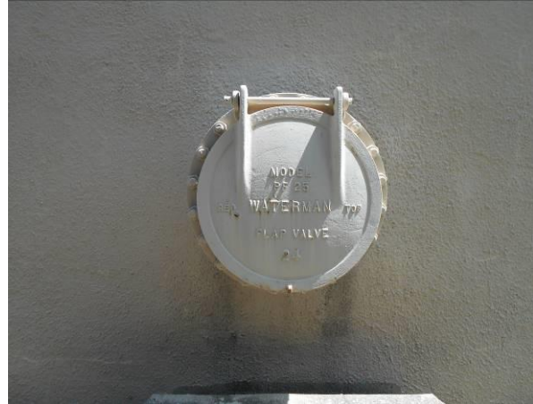
Photo No.38 – Overflow Flap Valve
