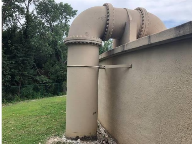
Photo No.27 – Inlet Pipe
