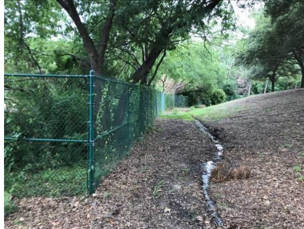
Photo No.24 - Chain Fence to be Replaced on East Side of Property
