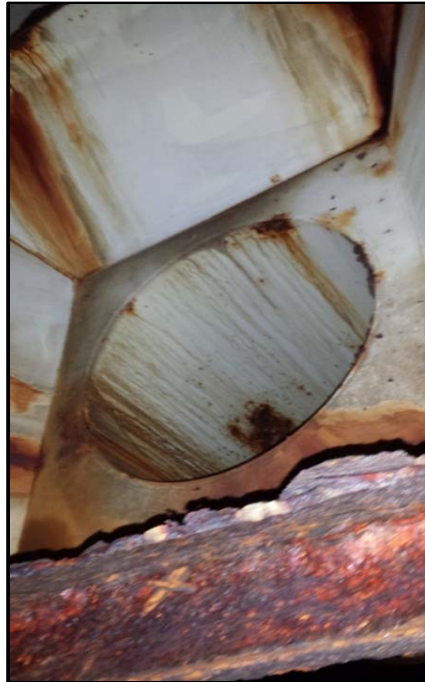
Photo 35 Overflow 1 - 24-inch Diameter Category: Operational
