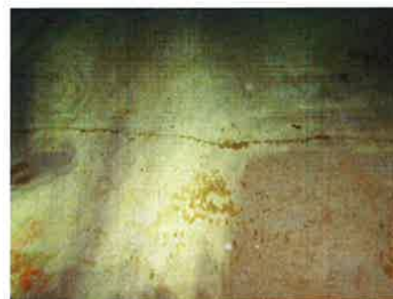
Crack in Tank Floor
