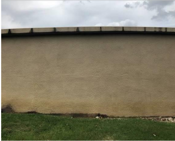
Photo No.7 - Staining
