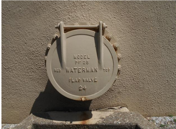
Photo No 37 – Overflow Flap Valve
