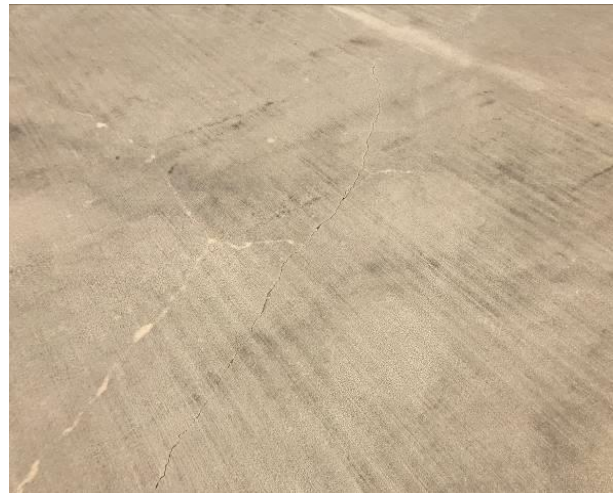
Photo No.2 - Cracking
