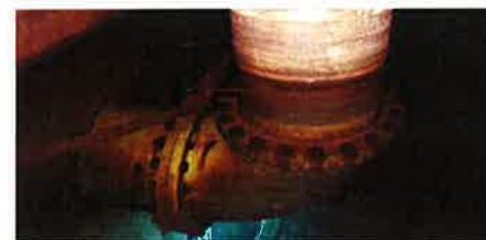
Corrosion of Bolts on Overflow Piping
