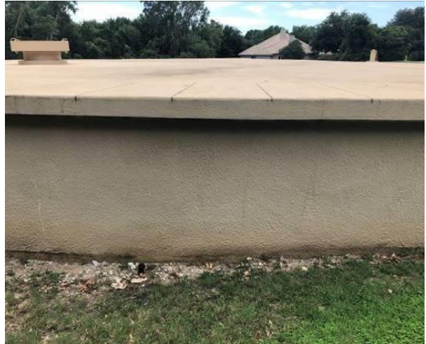
Photo No.8 - Cracking
