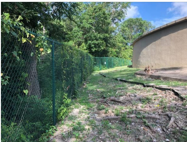
Photo No.43 – Moderate Erosion
