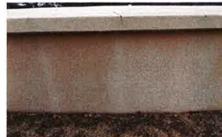
Exterior Wall Cracking
