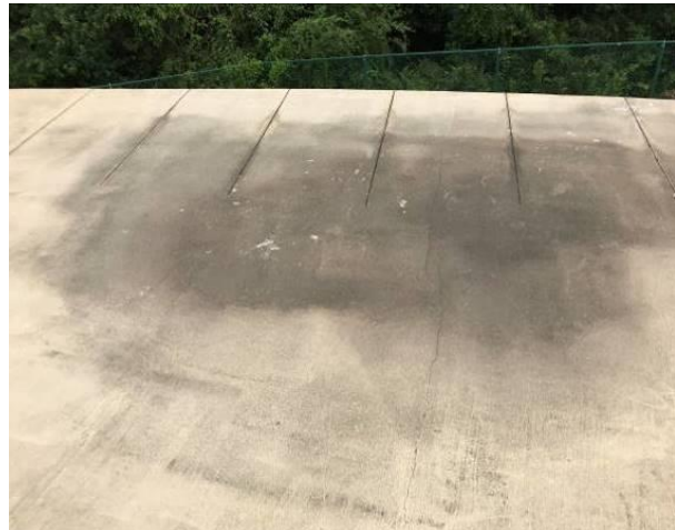
Photo No.4 - Water Ponding
