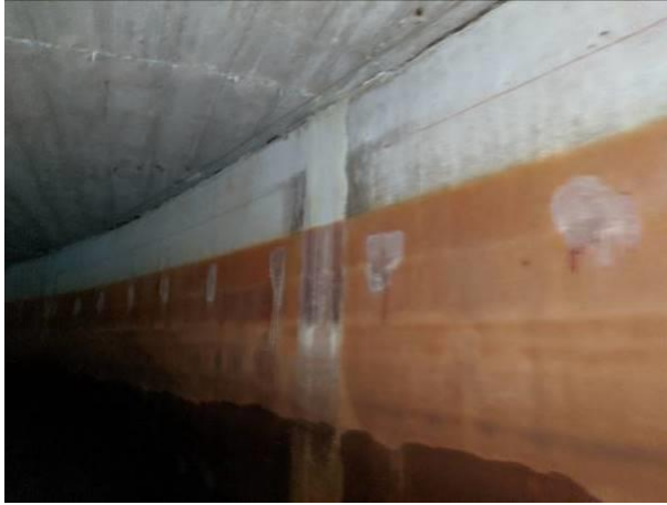
Photo No.15- Shell Wall Staining
