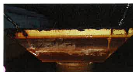
Corrosion of Steel Overflow Structure
