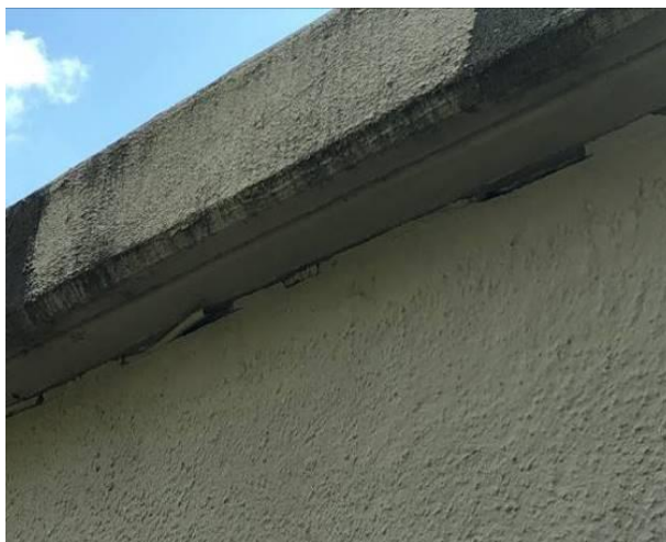
Photo No.5 - Grout Deterioration
