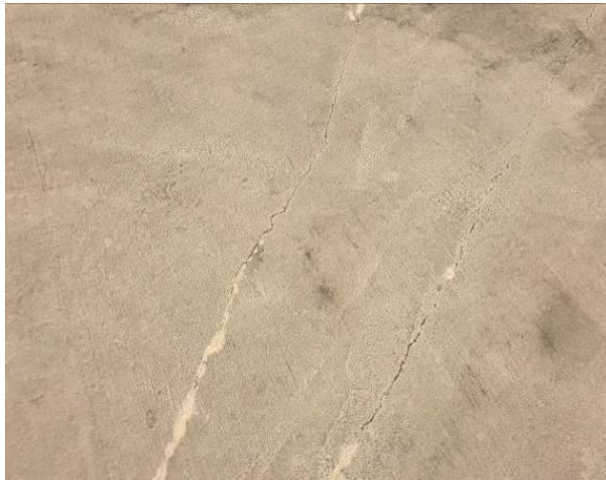
Photo No.3 - Cracking
