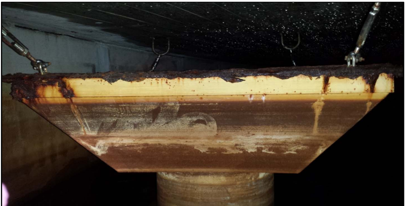
Photo 40 Overflow 2 - Weir Box - 4 feet 2 inches Wide by 4 feet 2 inches Wide Category: Operational
