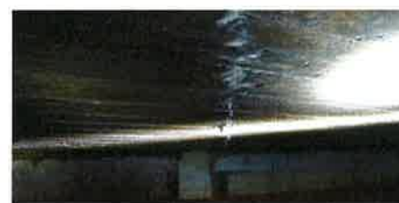
Interior Roof Cracking
