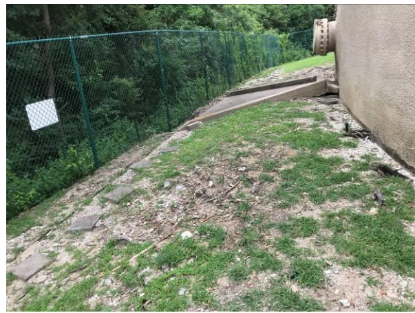
Photo No.44 – Moderate Erosion
