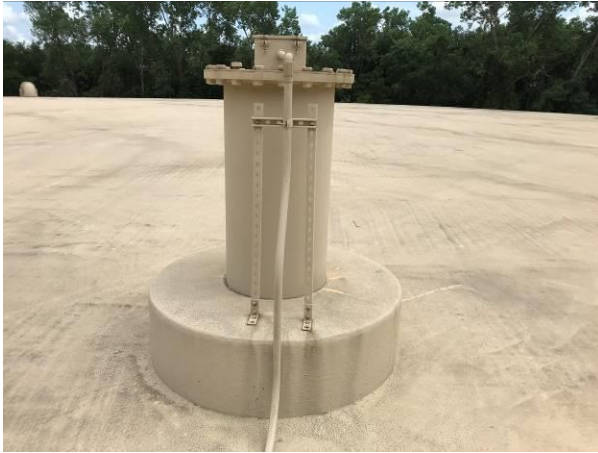
Photo No. 41 – Old Level Indicator
