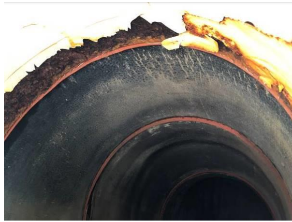
Photo No.32 – Overflow Pipe #2
