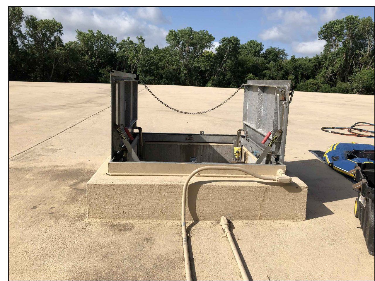
4 C11.0 EXISTING ROOF ACCESS HATCH REPLACE HARDWARE FOR DOOR SUPPORT AND INSTALL CONFINED SPACE SIGNAGE
