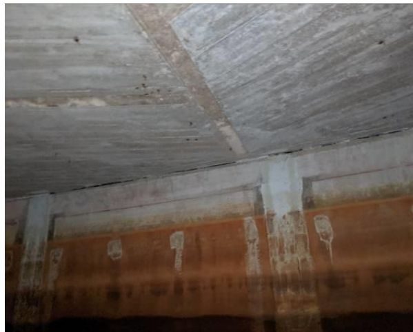
Photo No.14 – Grout Deterioration
