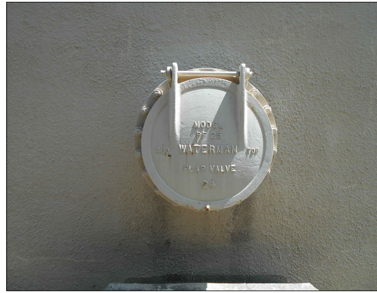
1 C11.0 EXISTING FLAP VALVE REMOVE AND REPLACE EXISTING FLAP VALVES PER CONTRACT DOCUMENTS ⚠️
