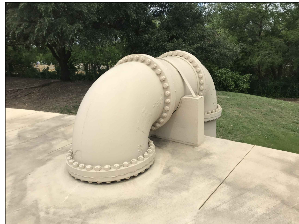
5 C11.0 EXISTING INLET PIPE REMOVE AND REPLACE THE SUPPORT PADS PER SPECIFICATION FOR THE INLET PIPE AND GROUT AS NECESSARY
