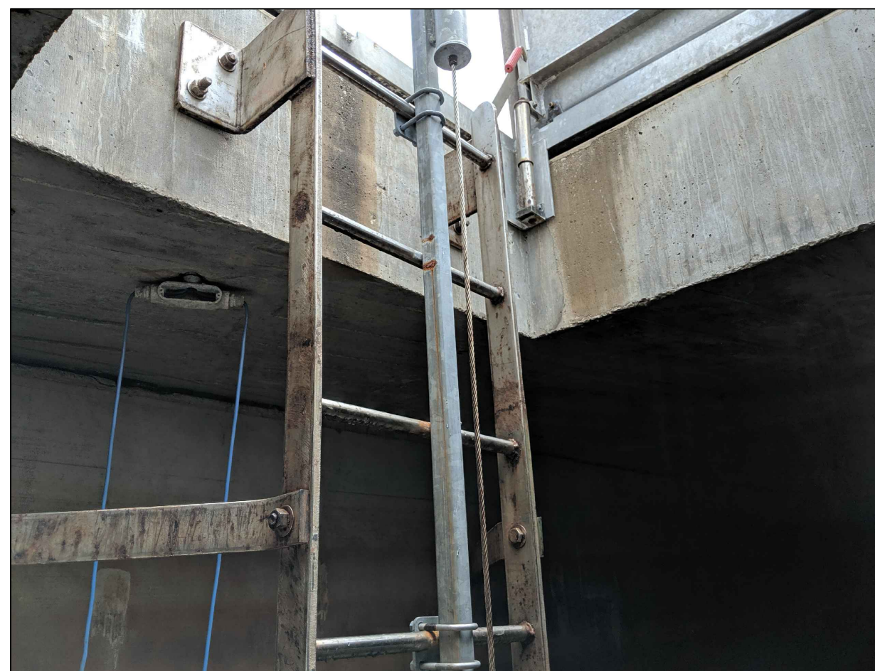
10 C11.0 EXISTING INTERIOR LADDER REMOVE EXISTING CAGE AND FALL PROTECTION SYSTEM. INSTALL NEW TS RAIL FALL PROTECTION SYSTEM
