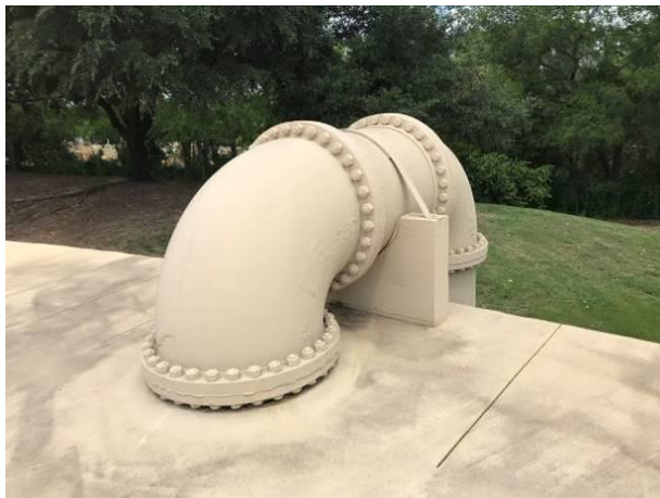
Photo No.25 – Inlet Pipe
