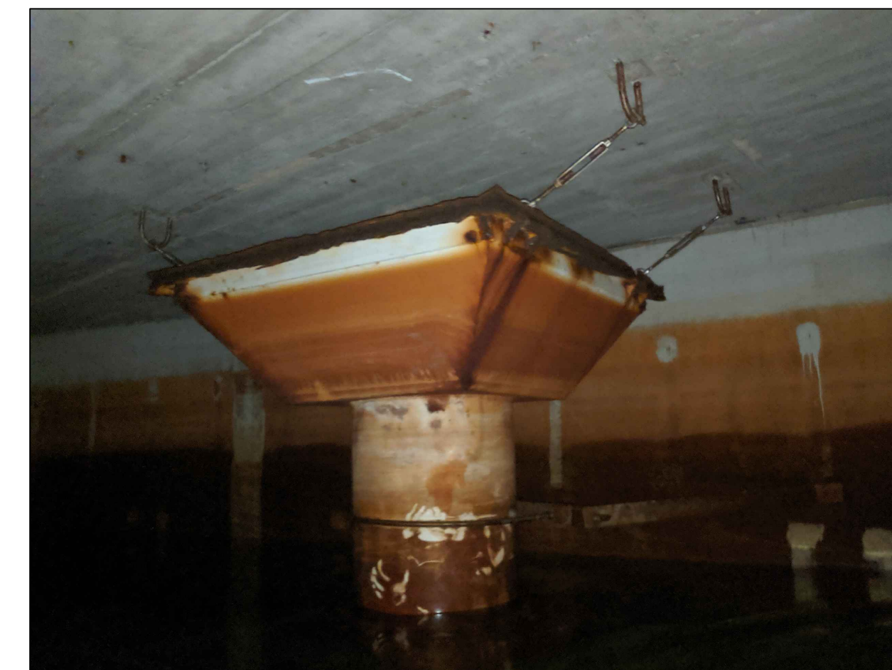
11 C11.0 EXISTING OVERFLOW WEIR REMOVE AND REPLACE THE EXISTING WEIR, PIPE AND SUPPORT PER CONTRACT DOCUMENTS ⚠️
