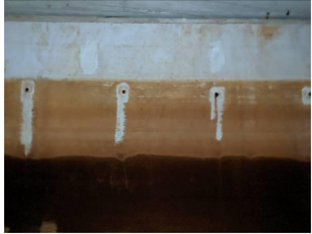
Photo No.16 - Exposed Rebar
