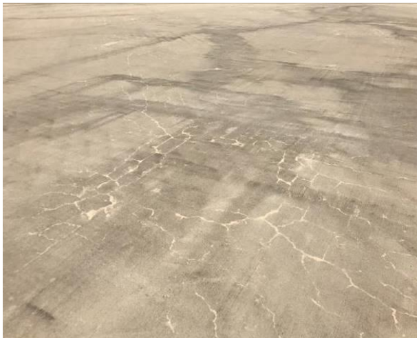
Photo No.1 - Cracking & Ponding
