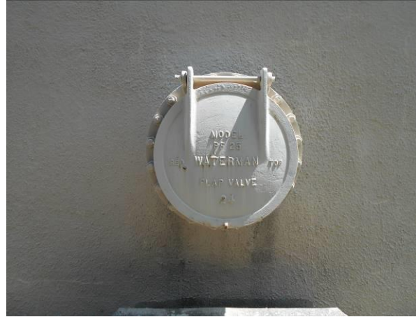
Photo No.38 – Overflow Flap Valve
