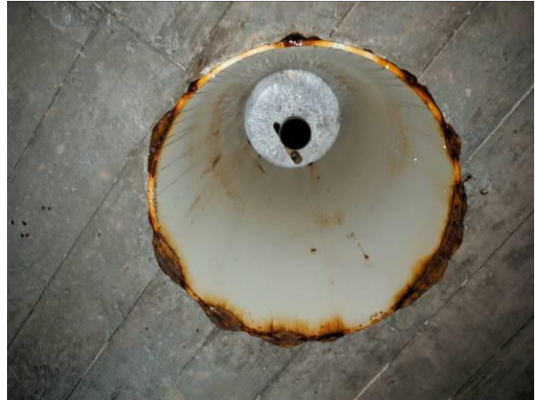
Photo No.42 – Old Level Indicator
