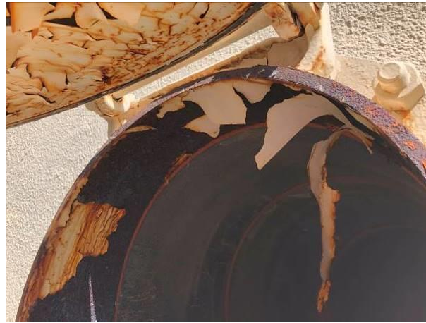
Photo No.30 – Overflow Pipe #1
