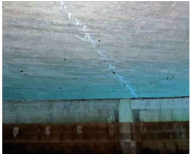
Photo No.10 - Efflorescence
