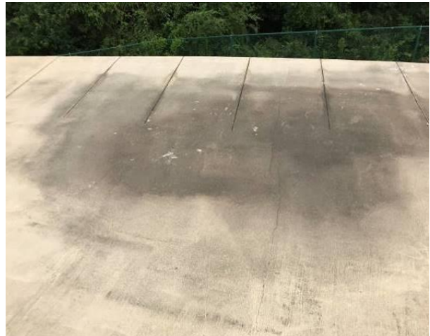
Photo No.4 - Water Ponding
