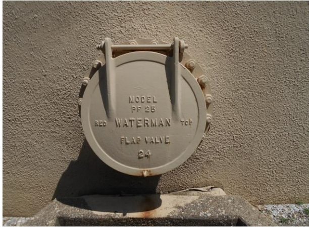
Photo No 37 – Overflow Flap Valve
