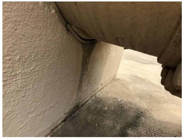
Photo No.26 – Inlet Pipe
