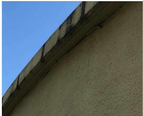
Photo No.6 - Grout Deterioration
