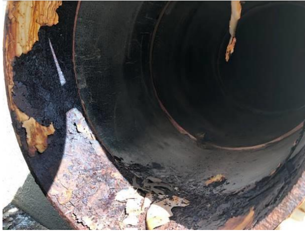
Photo No.29 – Overflow Pipe #1
