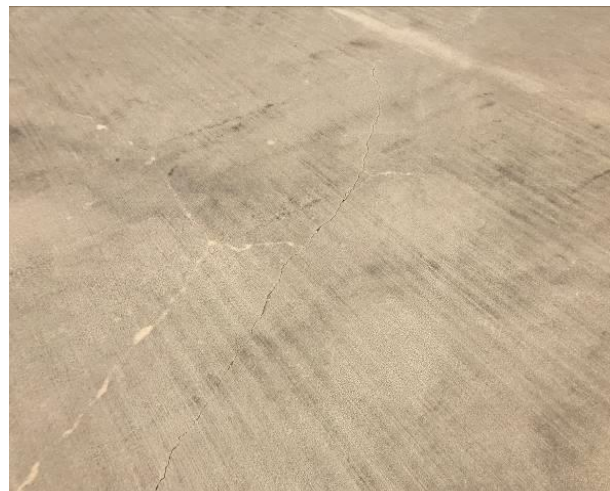
Photo No.2 - Cracking
