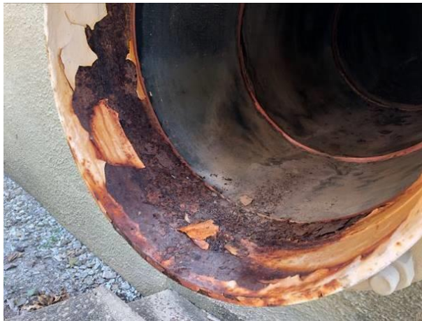
Photo No.31 – Overflow Pipe #2
