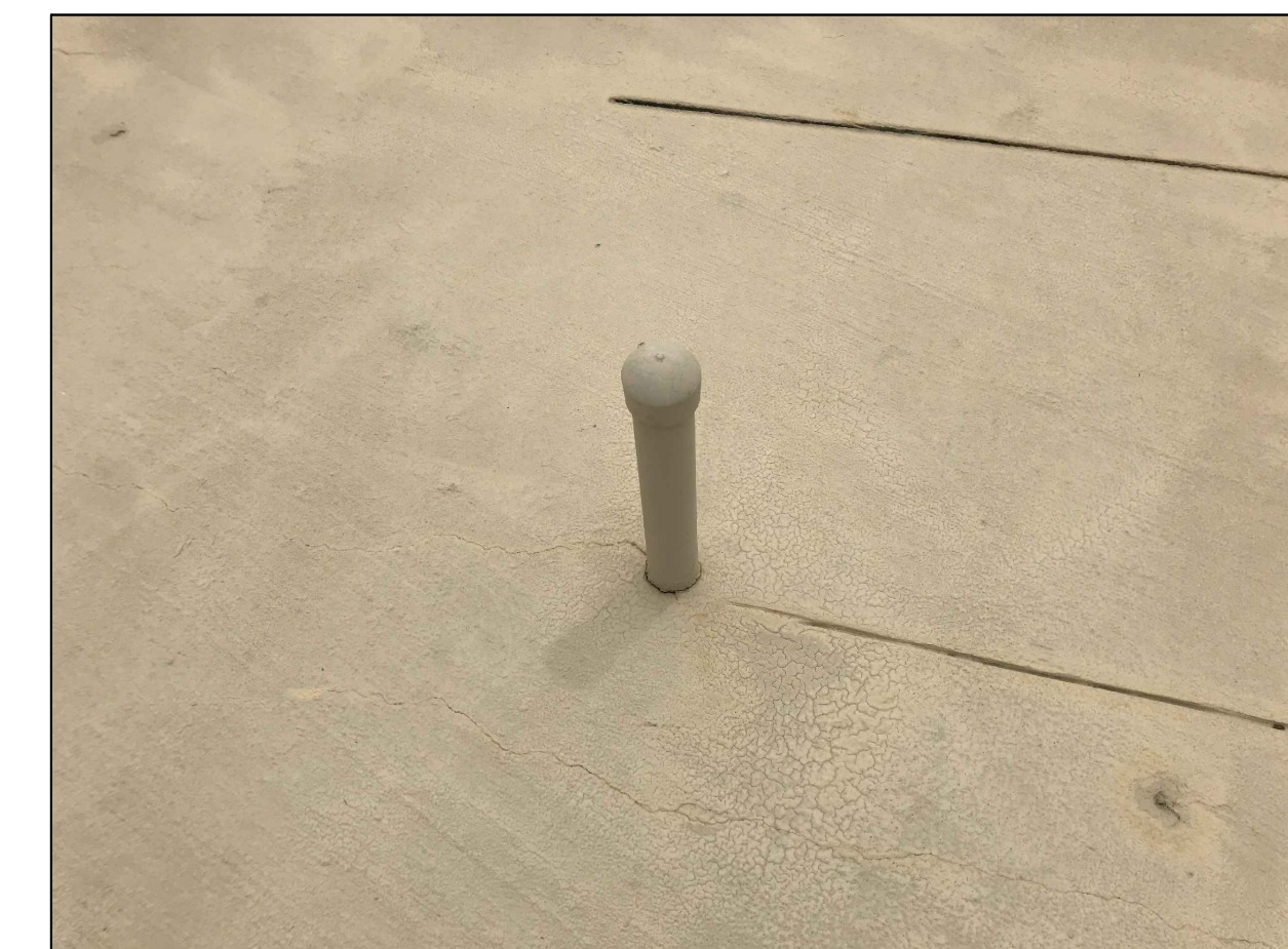
7 C11.0 EXISTING 2" PIPE SLEEVE REMOVE AND PATCH THE CONCRETE PER STRUCTURAL RECOMMENDATION
