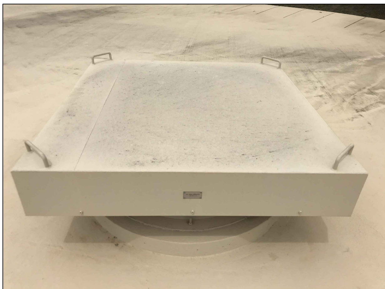
6 C11.0 EXISTING ROOF VENT BLAST AND RECOAT PER DIVISION 9. INSTALL CONFINED SPACE SIGNAGE
