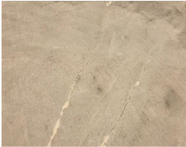
Photo No.3 - Cracking
