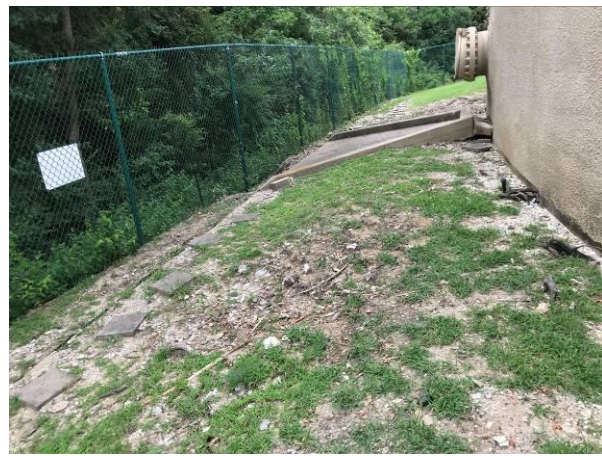
Photo No.44 – Moderate Erosion
