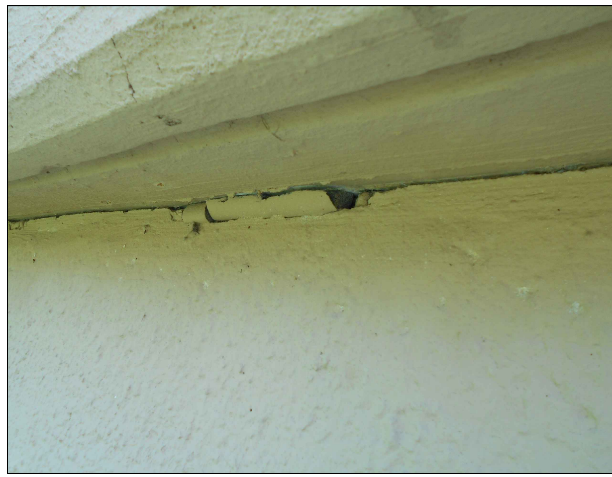
2 C11.0 EXISTING GROUT AT ROOF CONNECTION APPLY GROUT PER RECOMMENDATION IN SPECIFICATION
