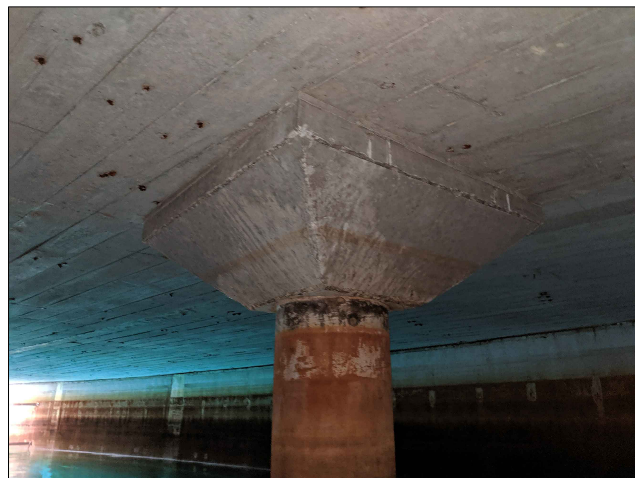
ROOF UNDERSIDE - RUST SPOT AND CRACKS (8) S4.0 NO SCALE
