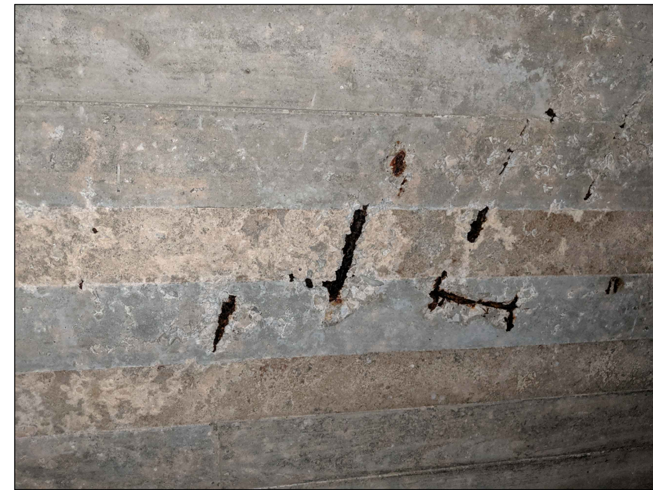
ROOF INTERIOR - EXPOSED & RUSTED REINF (6) S4.0 NO SCALE
