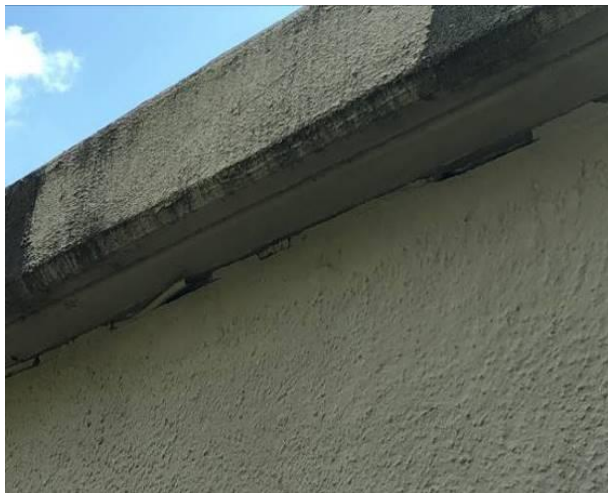
Photo No.5 - Grout Deterioration
