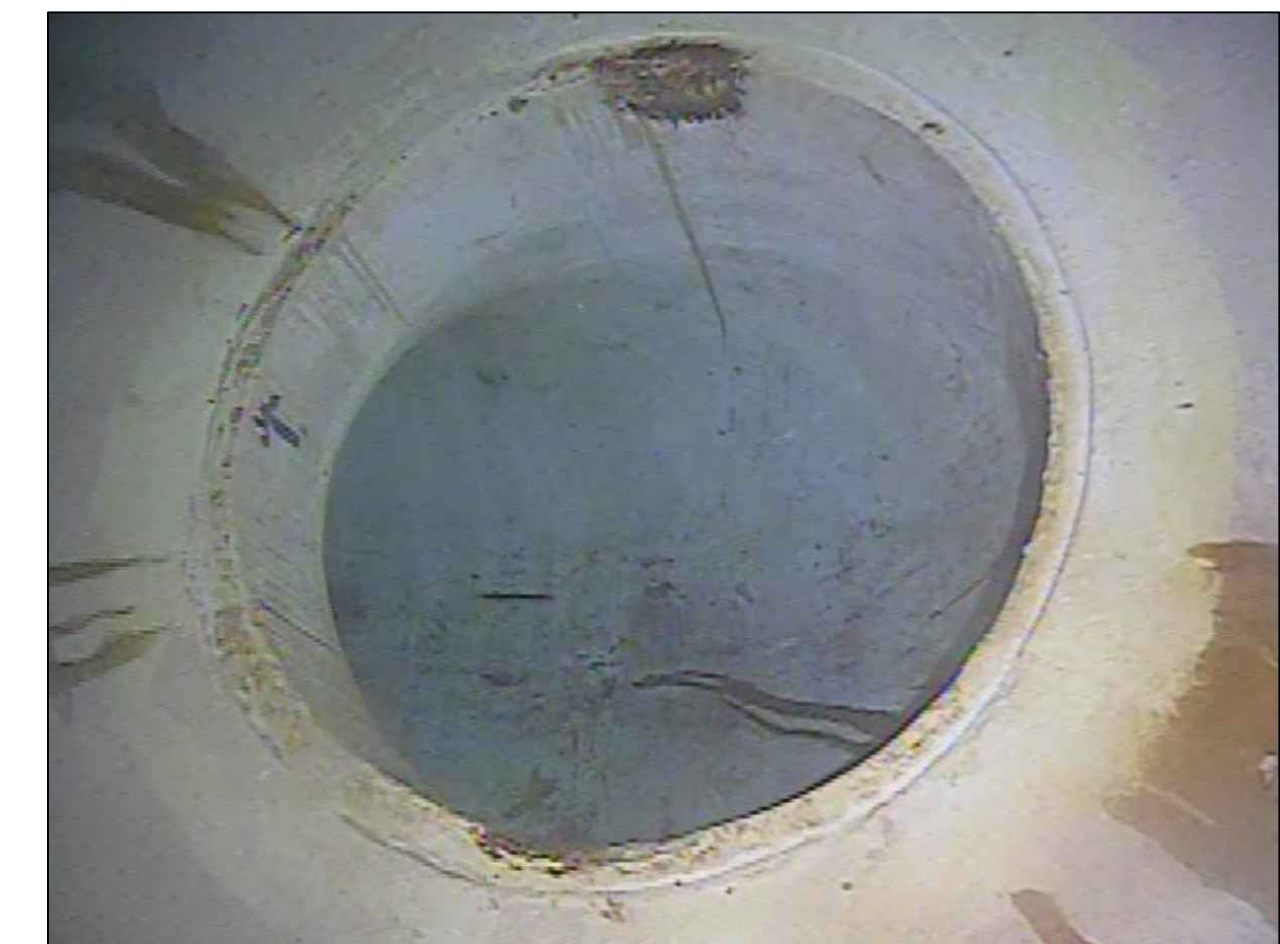
12 C11.0 EXISTING OUTLET PIPE BLAST AND RECOAT PER SPECIFICATION IN DIVISION 9. INSTALL NEW DEFLECTOR PLATE ⚠️
