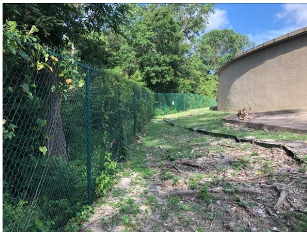
Photo No.43 – Moderate Erosion
