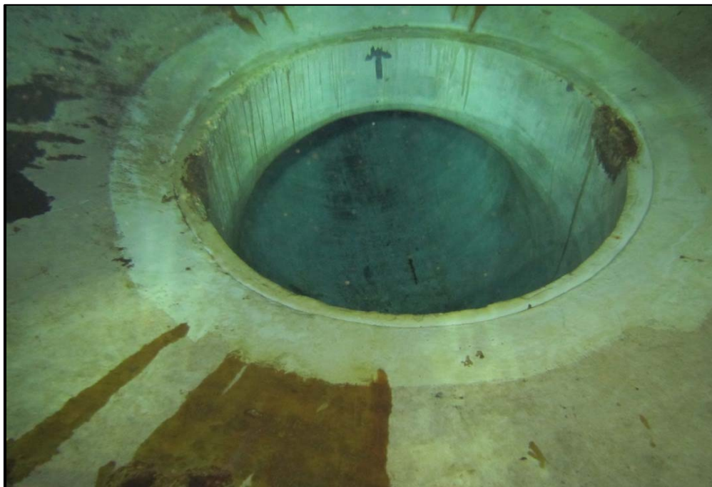
Photo 26 Outlet 1 - 42-inch Ductile Iron Category: Operational
