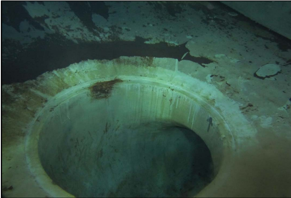
Photo 27 Outlet 2 - 42-inch ductile iron Category: Operational
