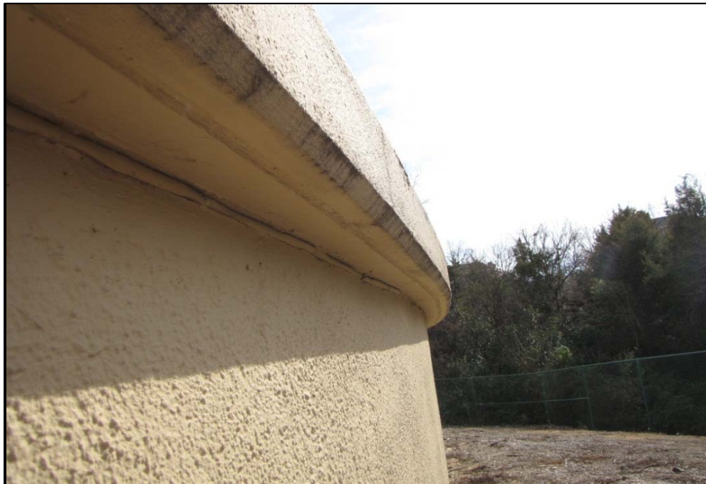
Photo 14 Shell Category: Structural
