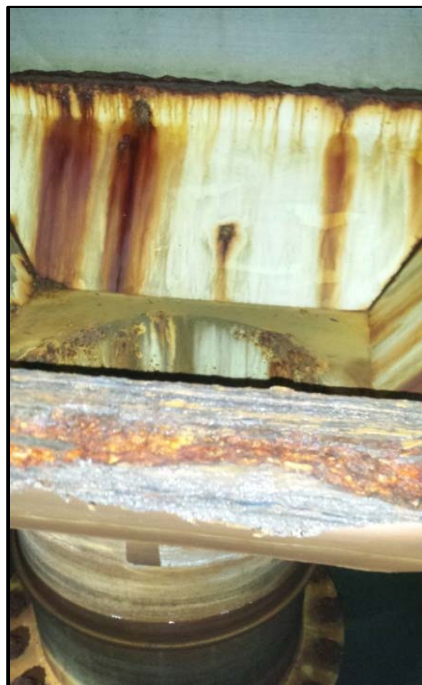
Photo 42 Overflow 2 - Weir Box - 4 feet 2 inches Wide by 4 feet 2 inches Wide Category: Operational
