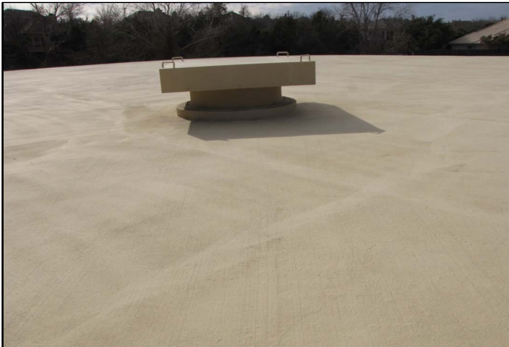
Photo 44 Vent - Fiberglass with 48-inch Opening Category: Operational
