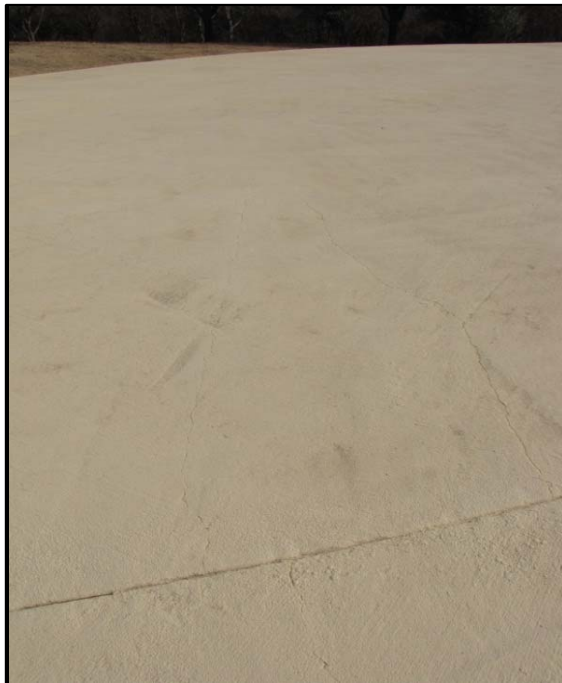
Photo 4 Roof - Construction Joint Category: Structural
