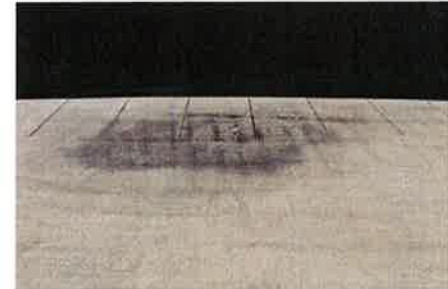
Ponding and Cracking in Exterior Roof
