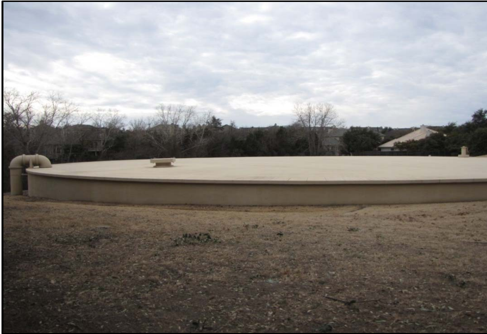
Photo 1 Roof of 206-foot interior diameter tank with slope of 0.25 inch per foot Category: Structural
