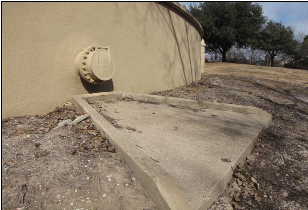
Photo 28 Overflow 1 - 24-inch Cast Iron Flap Valve and Concrete Splash Pad Category: Operational
