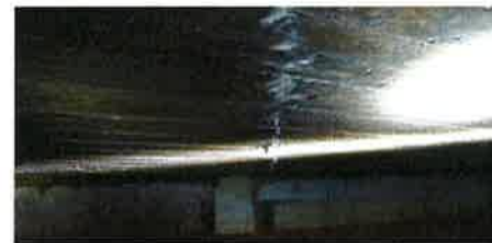
Interior Roof Cracking
