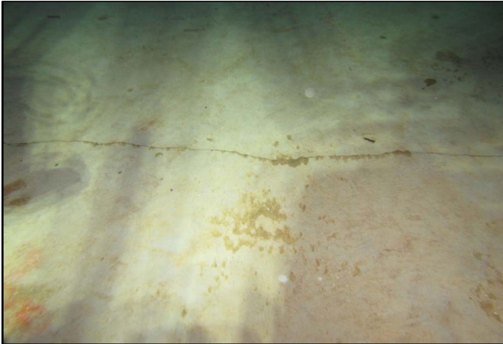
Photo 19 Interior Floor - Cracking was Observed Category: Structural
