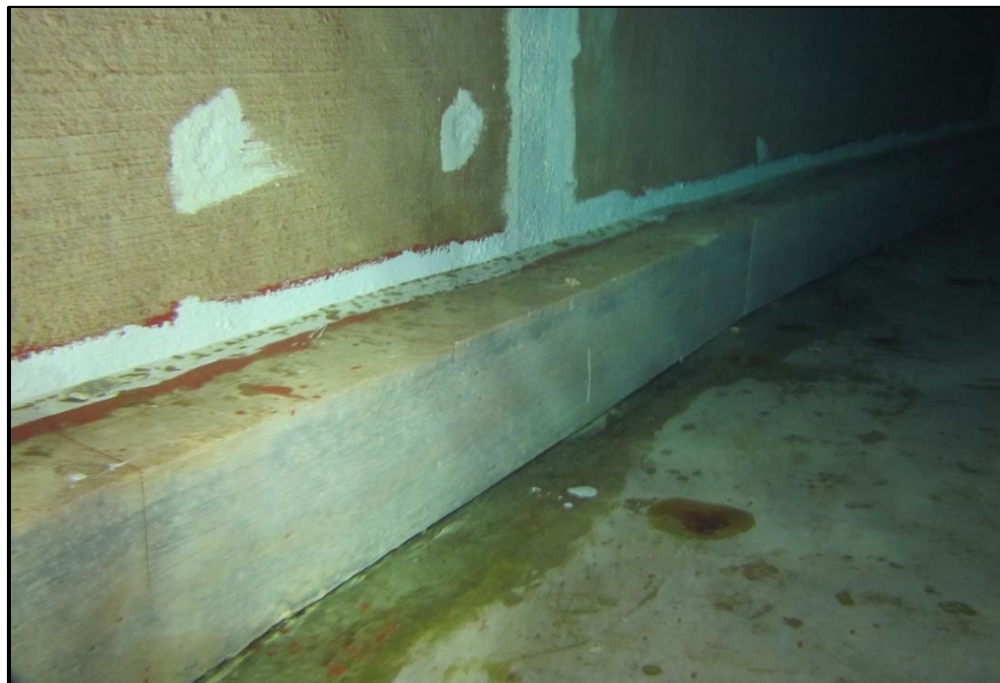
Photo 18 Water Stop Category: Structural
