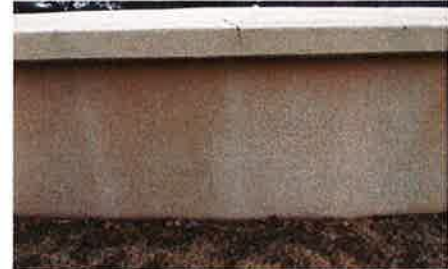
Exterior Wall Cracking
