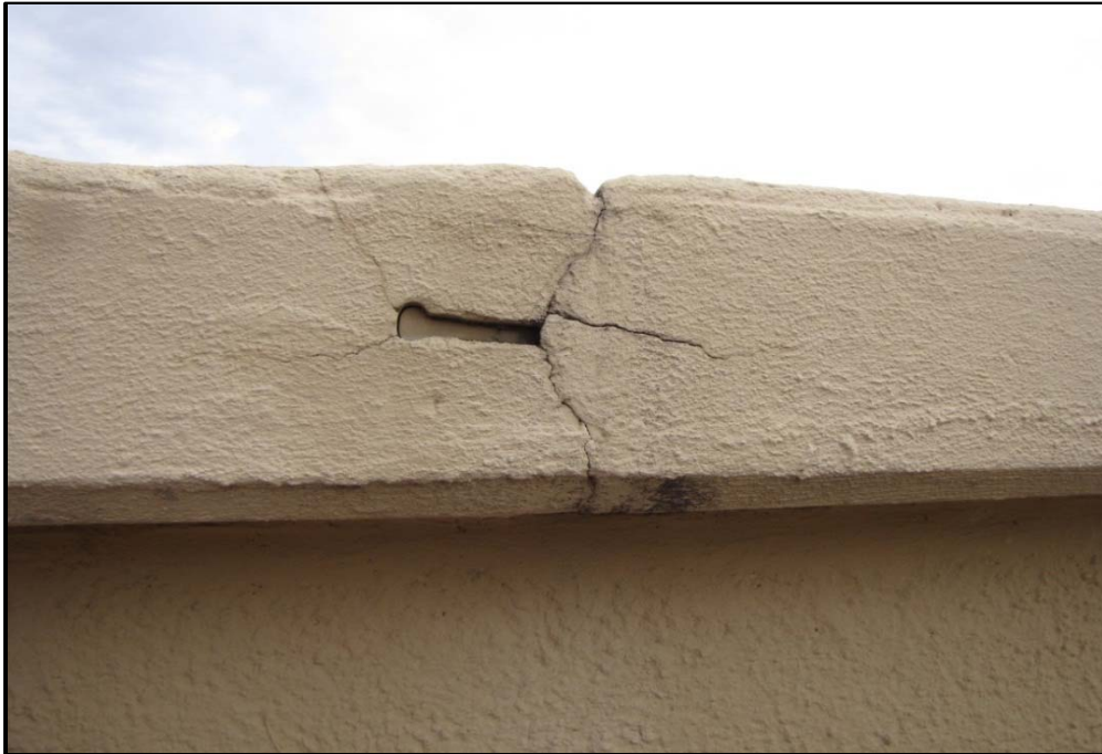
Photo 5 Roof - Severe Cracking Observed Category: Structural
