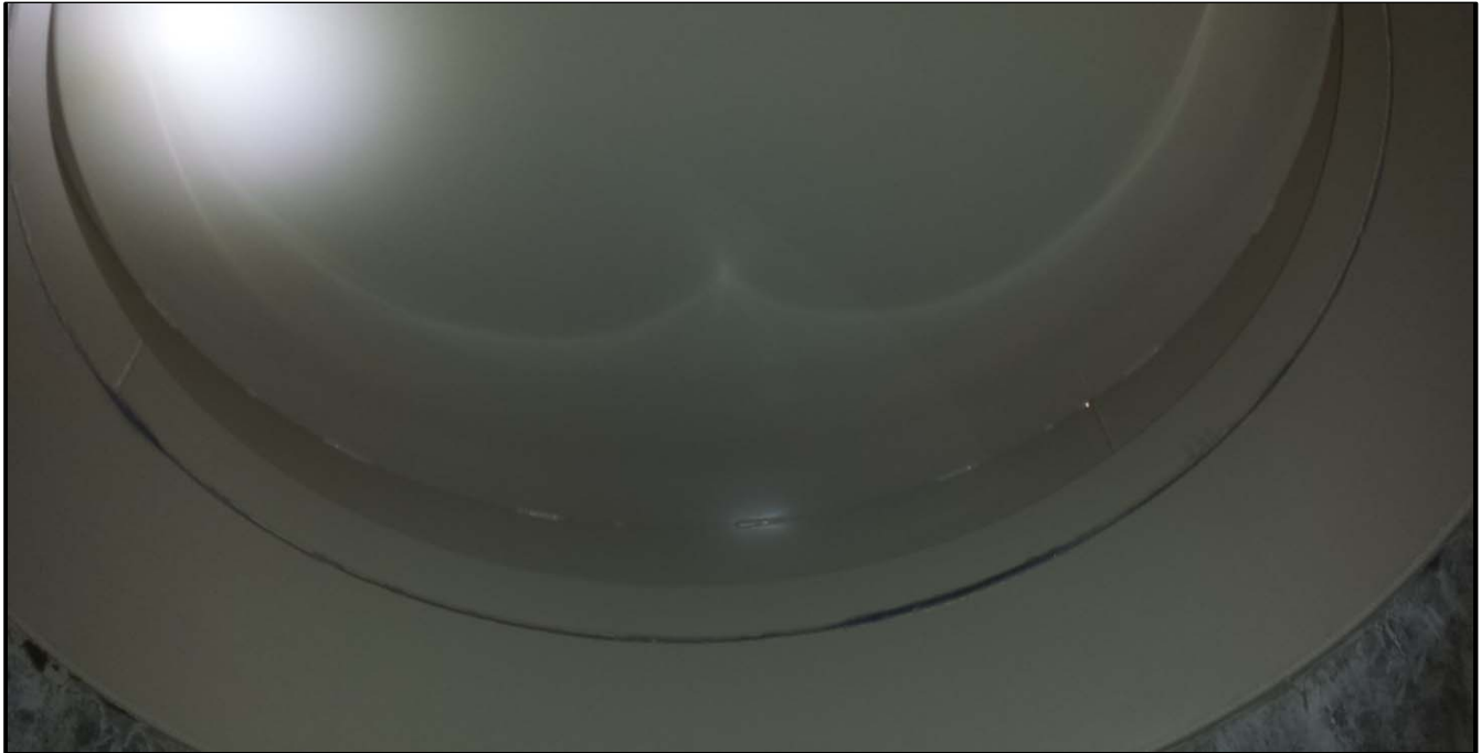
Photo 45 Vent - Fiberglass with 48-inch Opening Category: Operational
