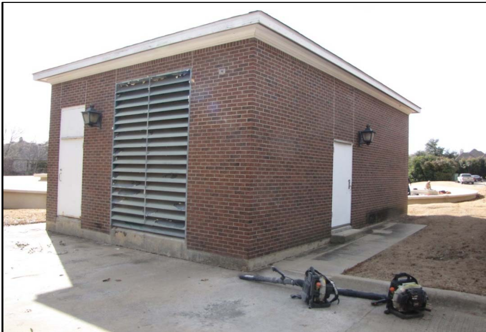
Photo 50 Control Building??? Category: Operational
