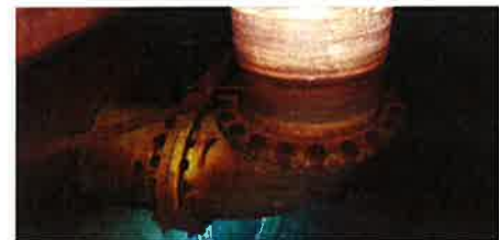
Corrosion of Bolts on Overflow Piping
