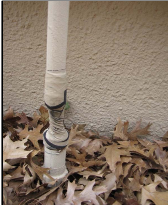
Photo 47 Electrical - Formerly for Sonic Level Transmitter Category: Operational
