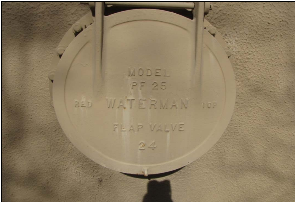
Photo 38 Overflow 2 - 24-inch Cast Iron Flap Valve Category: Operational
