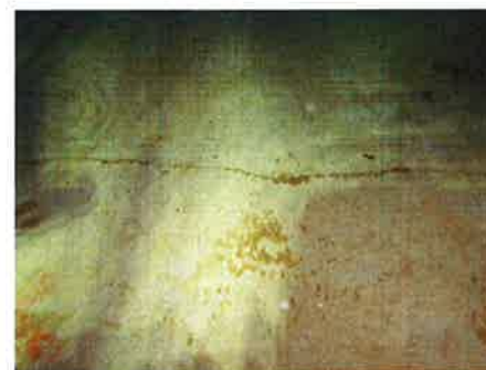
Crack in Tank Floor
