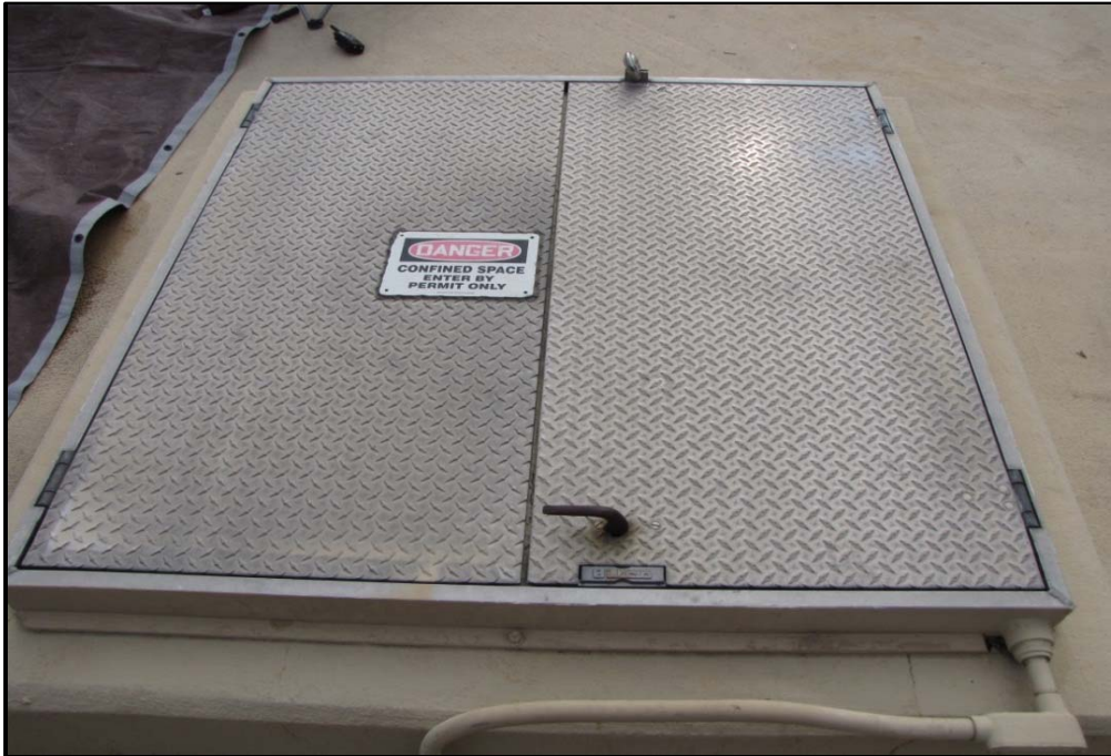
Photo 51 Roof Hatch - 4-foot x 4-foot Category: Safety & Security
