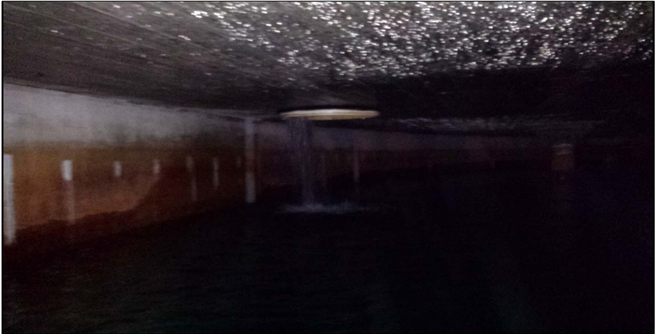
Photo 25 Interior Inlet - 36-inch Ductile Iron Category: Operational
