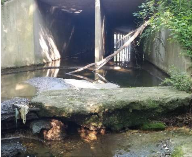
Photo 13: Scour and Undermining
