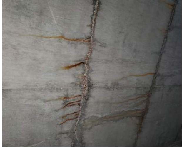
Photo 18: Transverse Crack in Top Slab with Efflorescence
