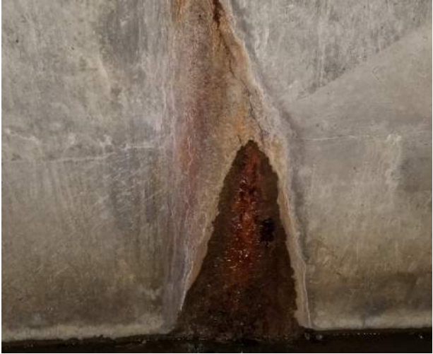
Photo 17: Vertical Crack in Wall With Efflorescence Build-Up
