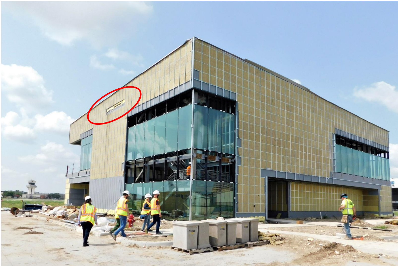
Changes to the scuppers on the south side of the building (September 25, 2020).
