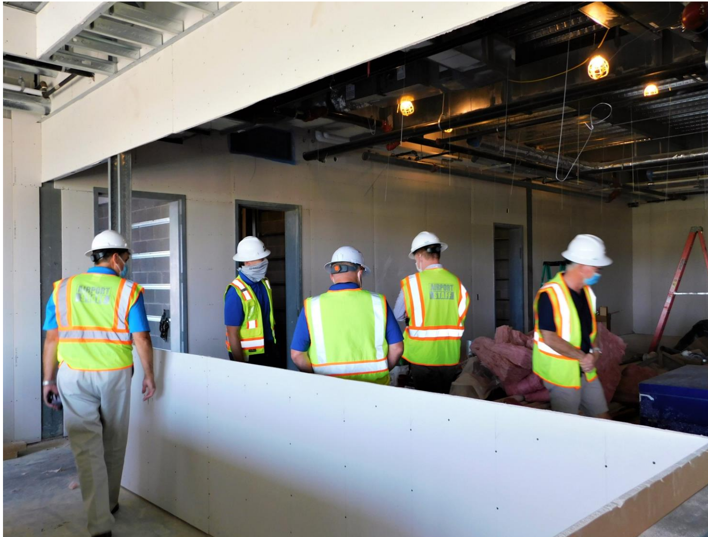
Area of changes to the wall support framing viewed from the post-processing area (September 25, 2020).
