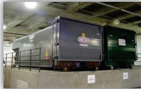
35 yard trash & recycle compactors in dock area
