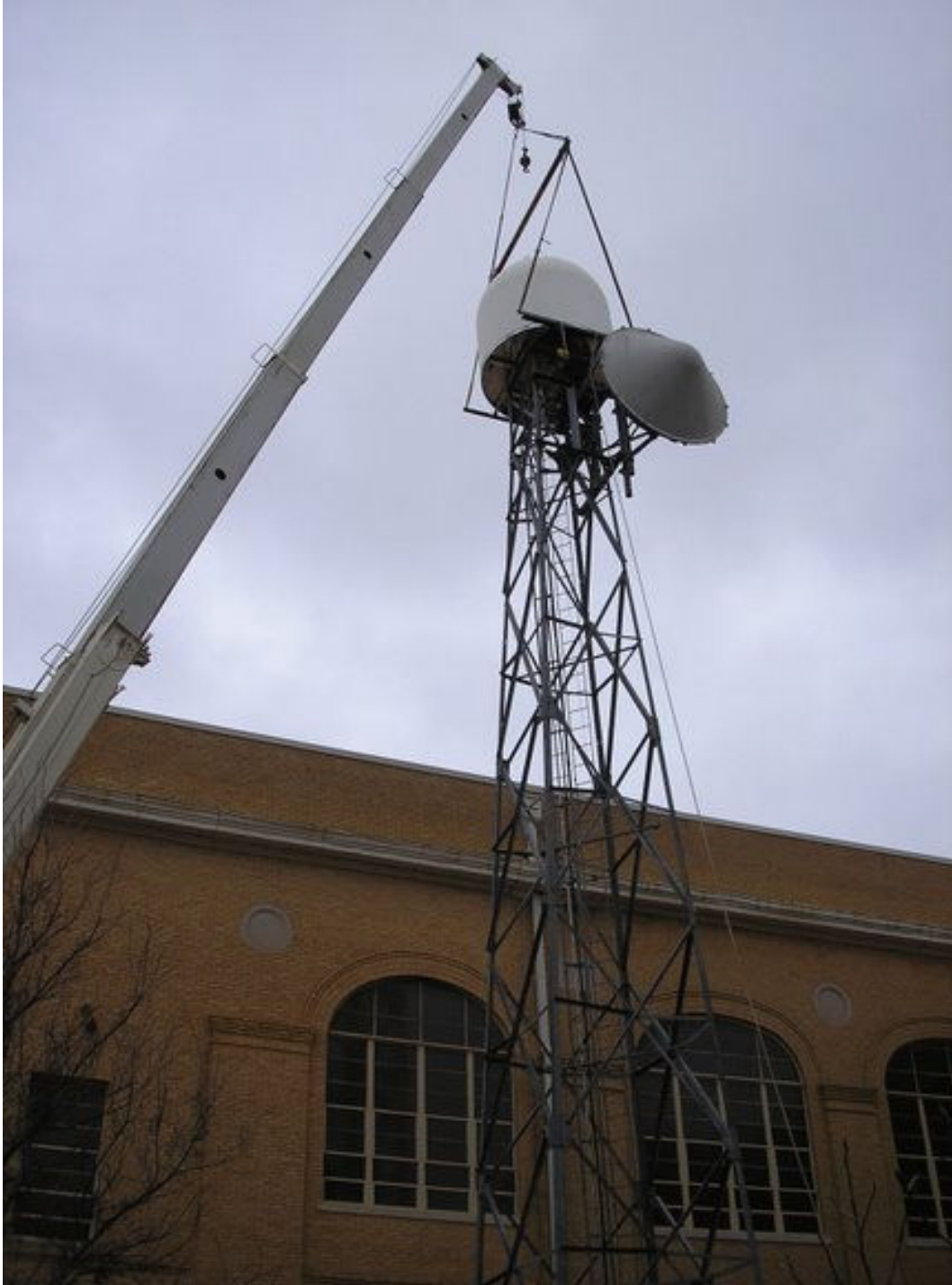
Figure 17 - A square pyramid tower adjacent to an existing building with a microwave antenna mounted alongside for communications.
