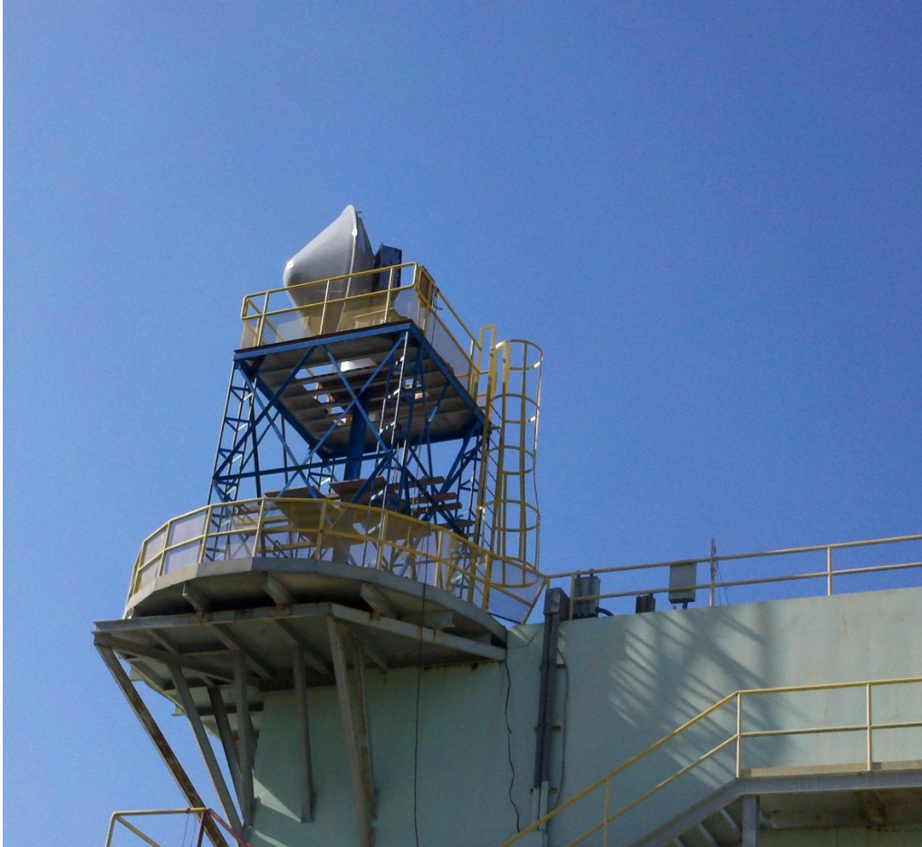
Figure 25 – Radar mounted on roof platform to clear surrounding structures. Rest of radar computing and networking equipment is housed inside the building.
