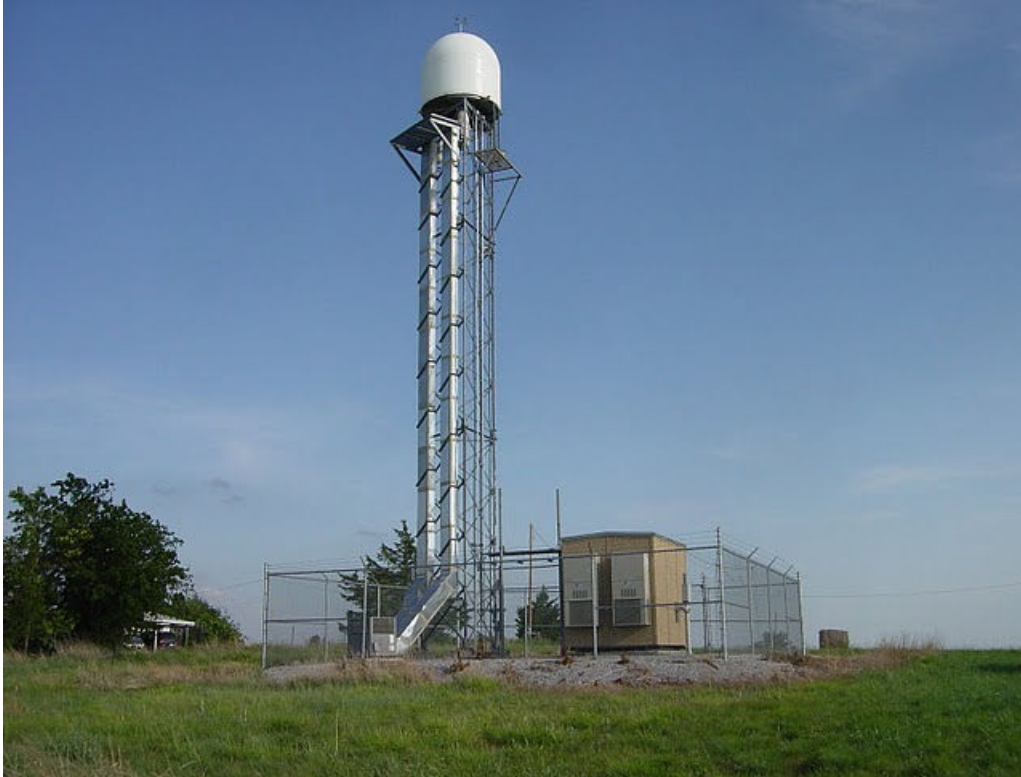
Figure 30 - Complete tall tower installation with prefabricated shed
