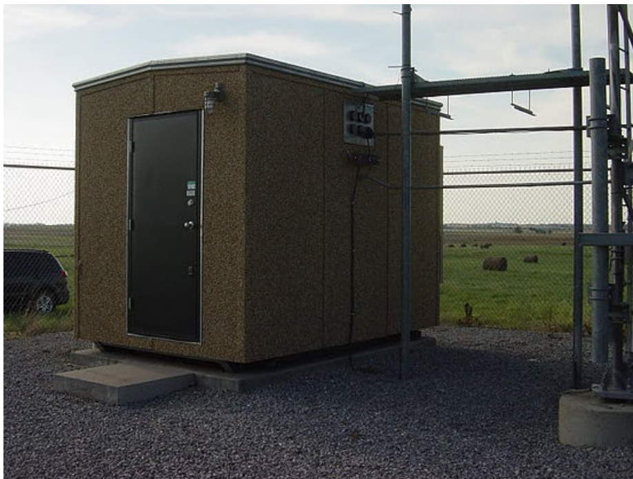
Figure 27 - Cable pass-through to tower base and equipment shed
