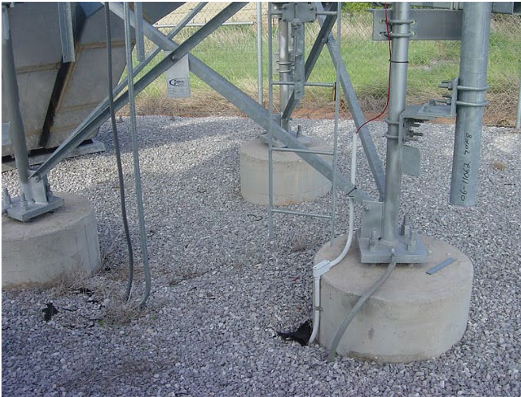
Figure 14 - Triangular tower mounts, with cable conduit and grounding
