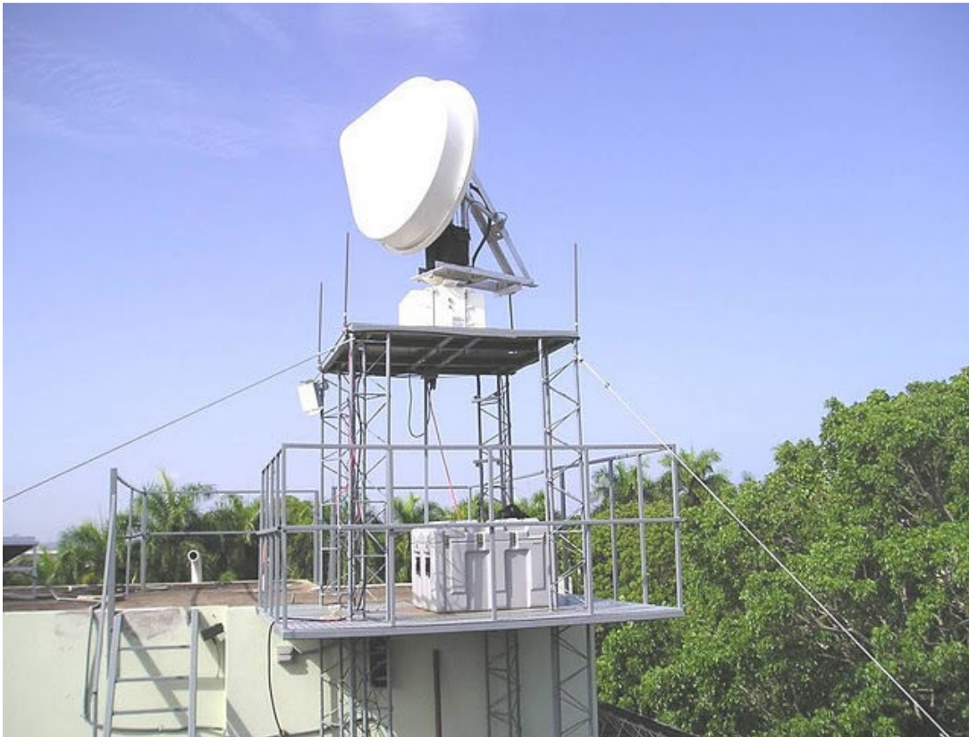
Figure 24 - Radar mounted on a small platform, elevated off a rooftop. Weatherized computer equipment housing box seen below
