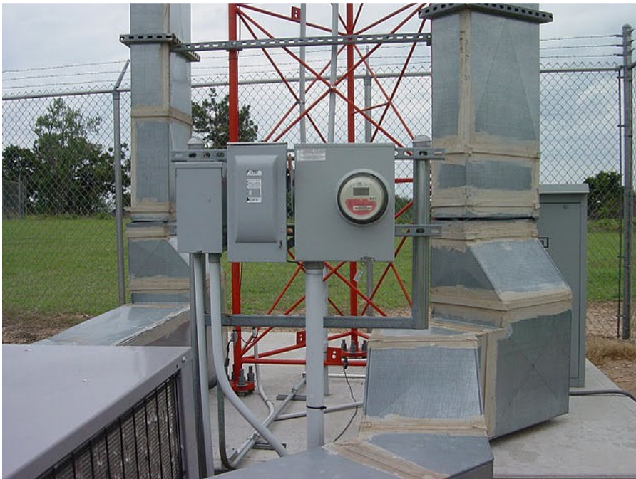
Figure 11 - Breaker box, Meter, Ductwork
