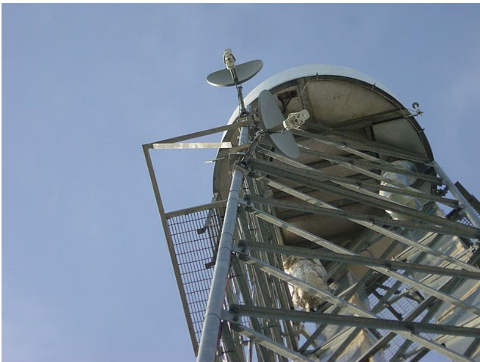
Figure 23 - Wireless radio antennas mounted to tower
