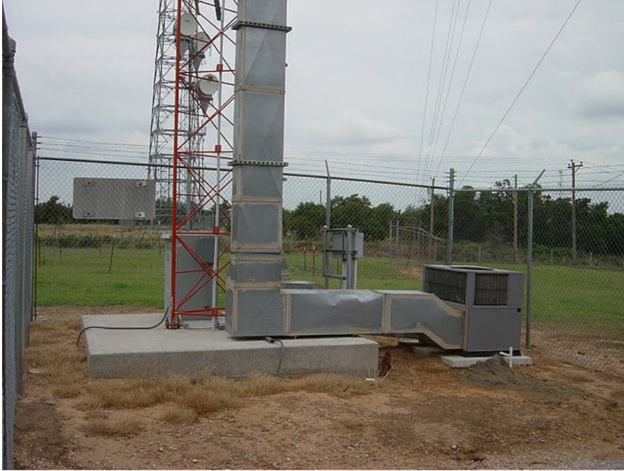
Figure 10 - HVAC unit, Ductwork, Security fence
