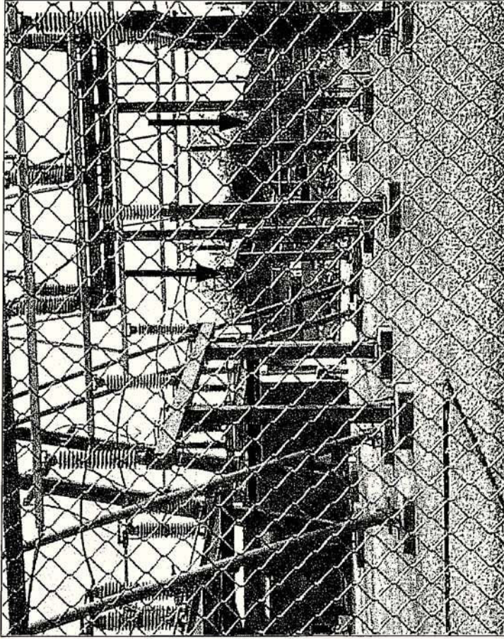
Substation in Grand Prairie, with residential in background (arrows).
