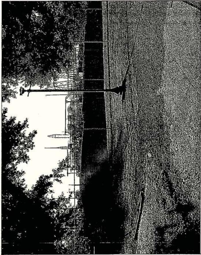
Standard substation on Greenville Avenue.
