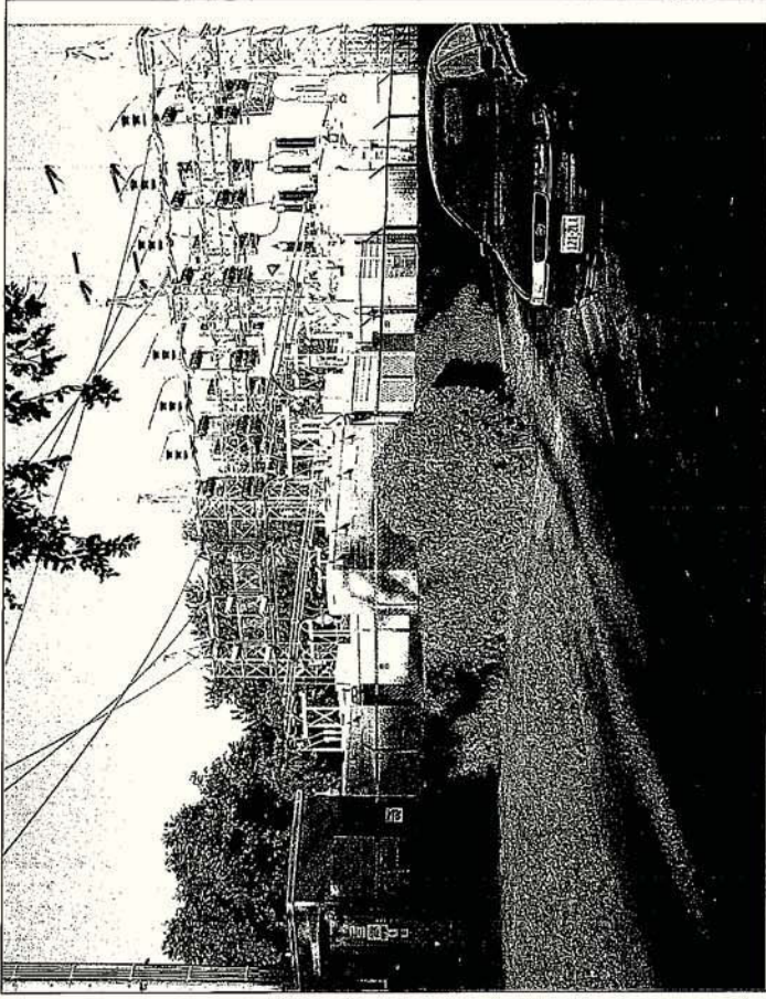
University Park substation homes across street valued at over $500,000.
