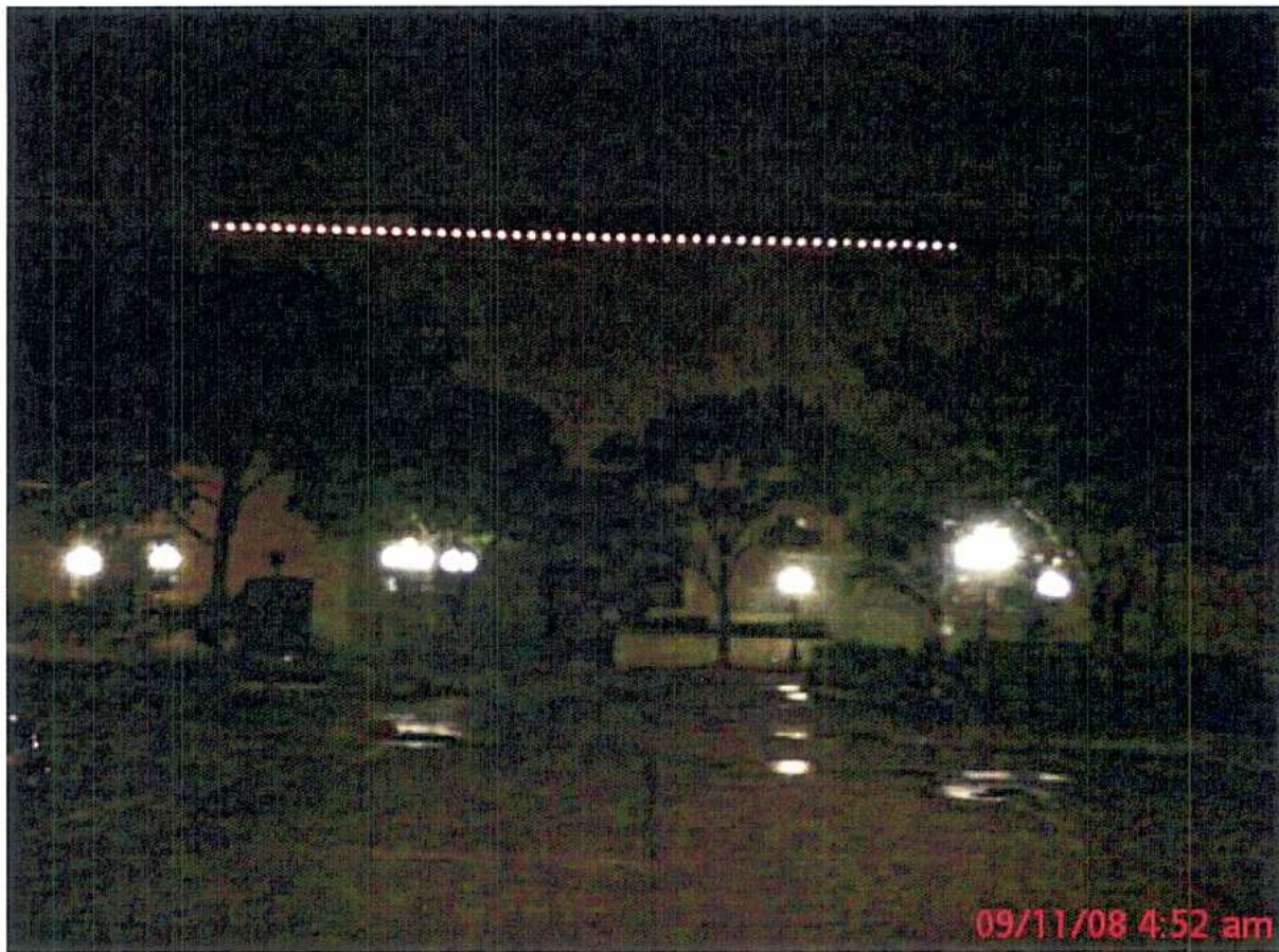
Sample Light installation located on South East corner of Bed Bath & Beyond building. 2 nd Level
